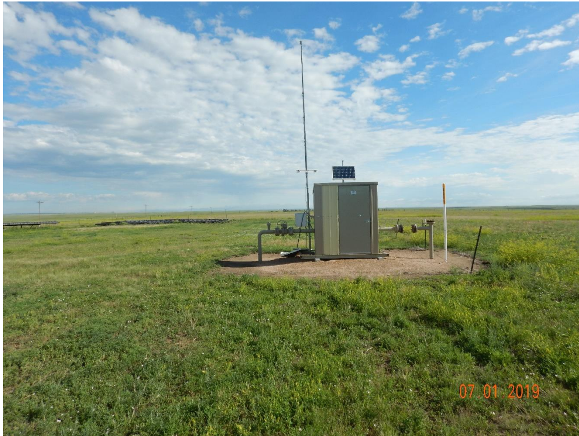
Photo 12: Photo taken from the east end of the location, facing north. Photo shows equipment has not been removed from the location, or reclamation conducted.
