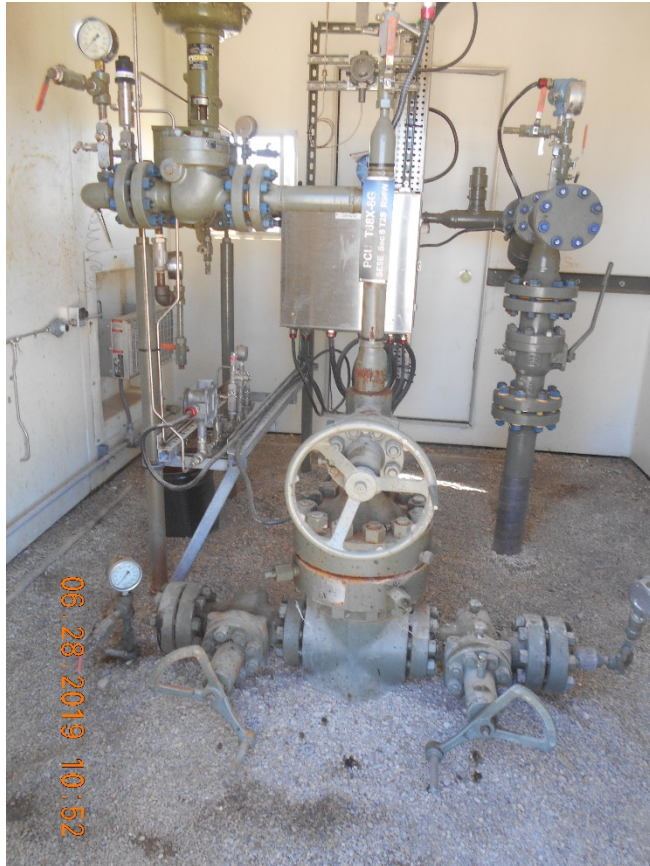
Injection wellhead inside housing
