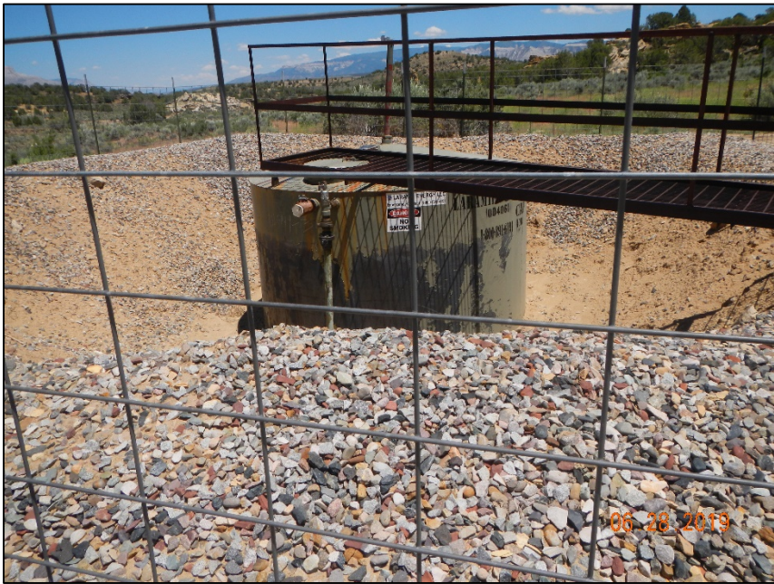
Photo # 3 Photo of Tank Battery
