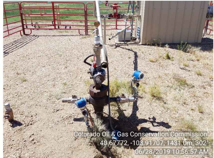
Photo #2 Lilli Unit 8-12 UIC - Injection Well Shut-In | SI Not Injecting
