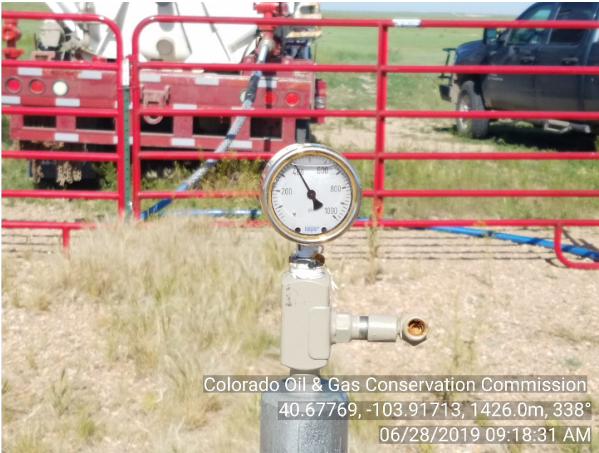
Photo #3 Lilli Unit 8-12 UIC - Injection Well Tbg. Press: 400# Shut-In | SI Not Injecting
