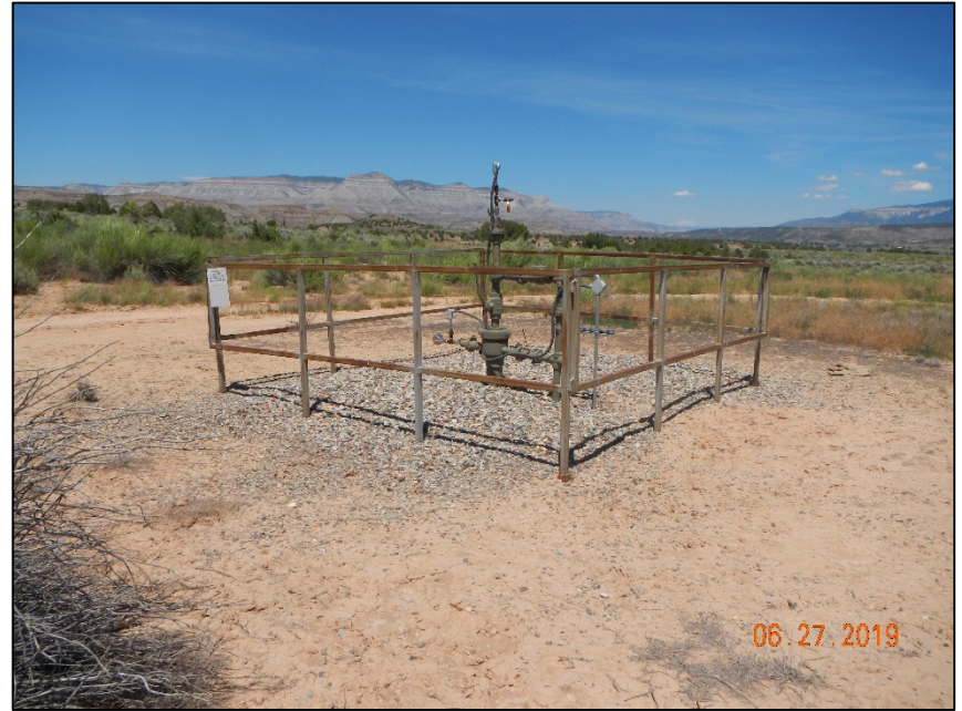
Photo # 4 Photo of Wellheads.
