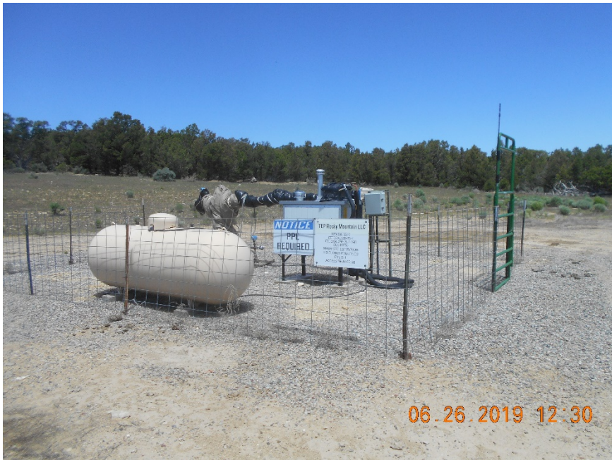
Injection wellhead & line heater
