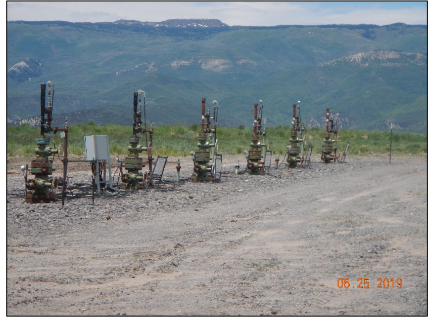
Photo # 4 Photo of Wellheads.
