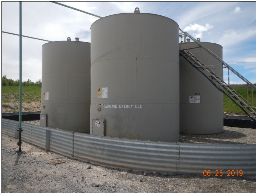
Photo # 3 Photo of tank Battery
