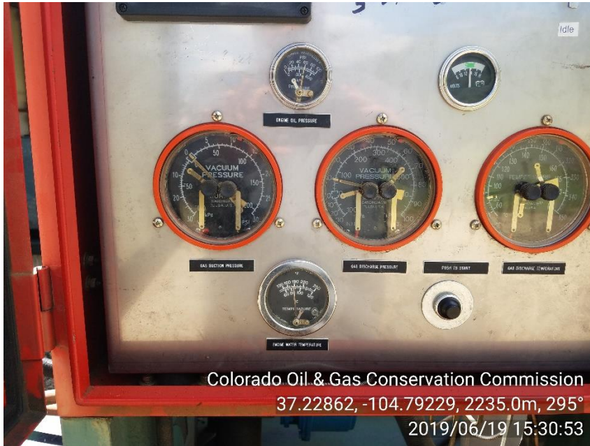
PHOTO 5: Vacuum pump observed on well without COGCC approval. Provide COGCC with documentation showing approval of use of vacuum pump. CA DATE 7/6/19.
