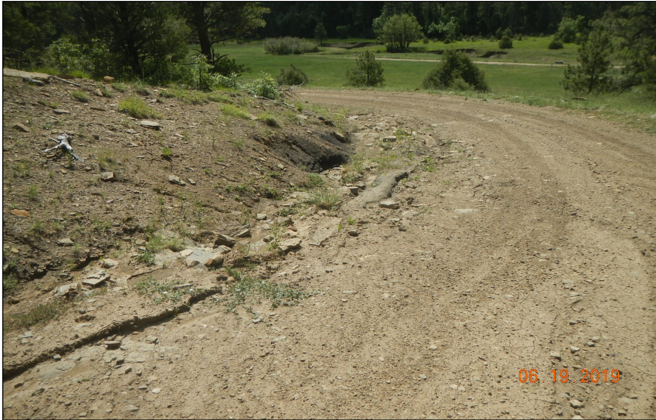
Photo 2. There is erosion occurring down the road and no BMP's are installed.
