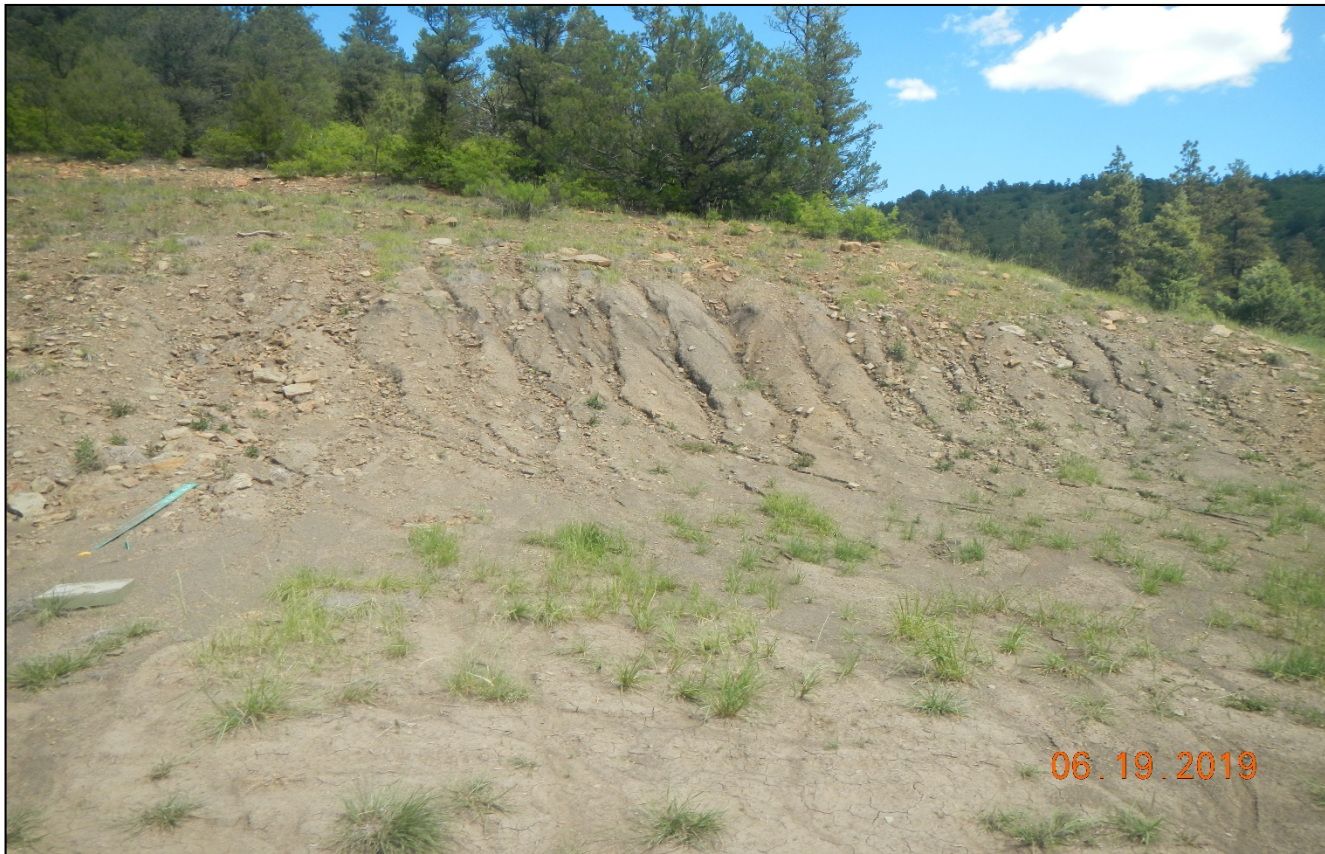
Photo 4. There is signs of erosion occurring from the cut slope.
