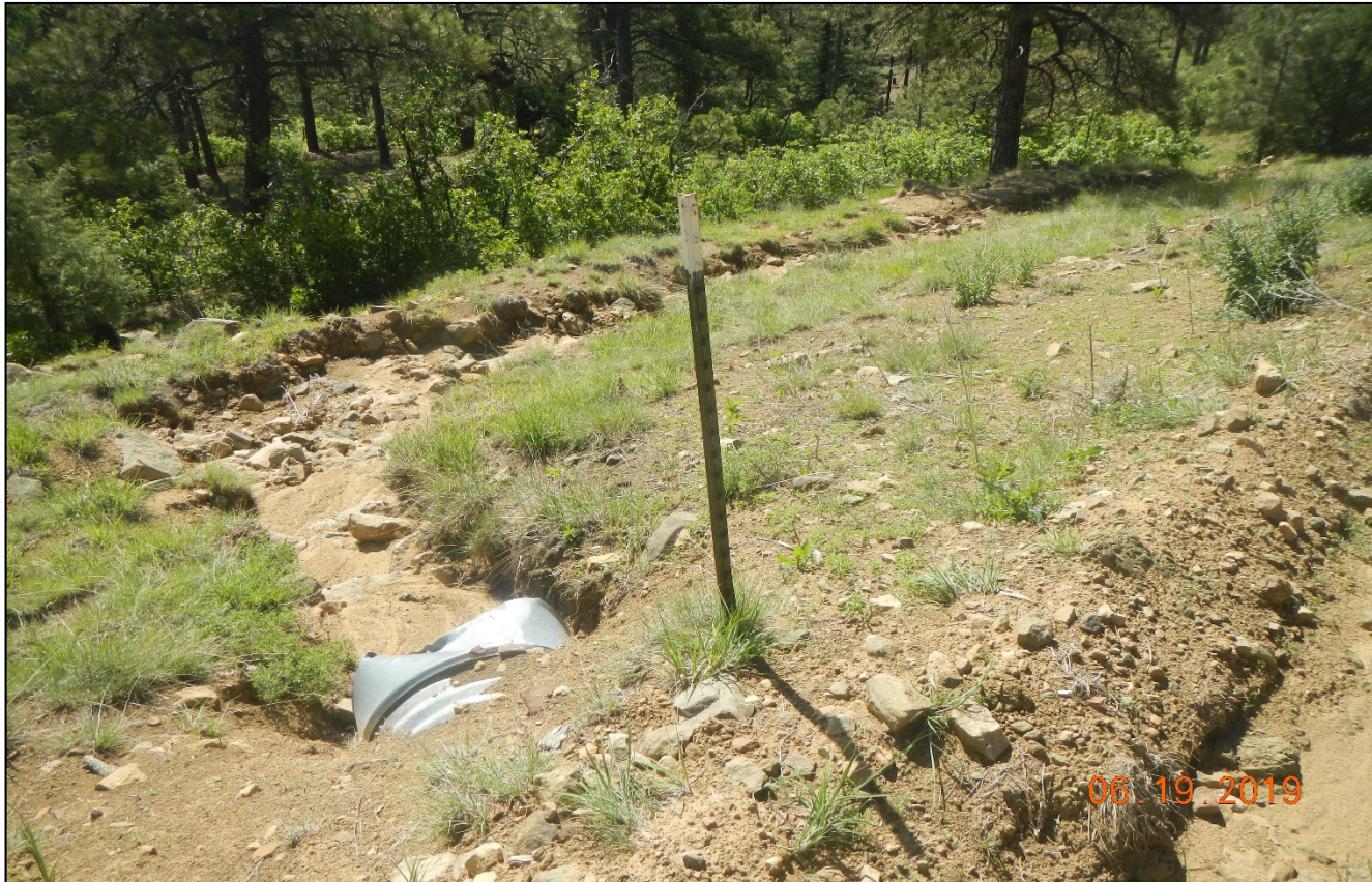
Photo 1. The outlet culvert at the location has no BMP's to prevent erosion.
