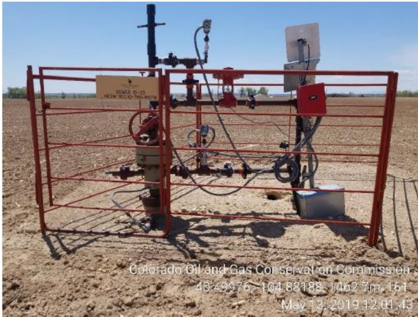
Photo 1: PREVIOUS photo of NO emergency contact # on sign
