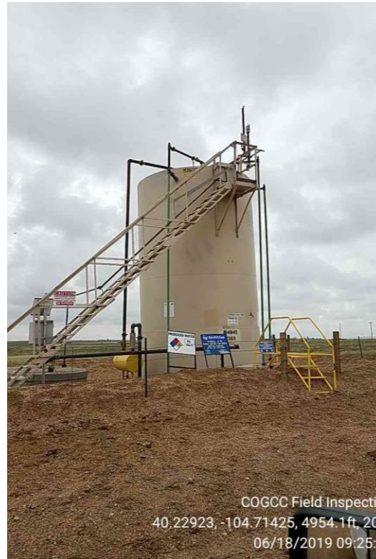
Photo 2 Remote Battery South of Well
