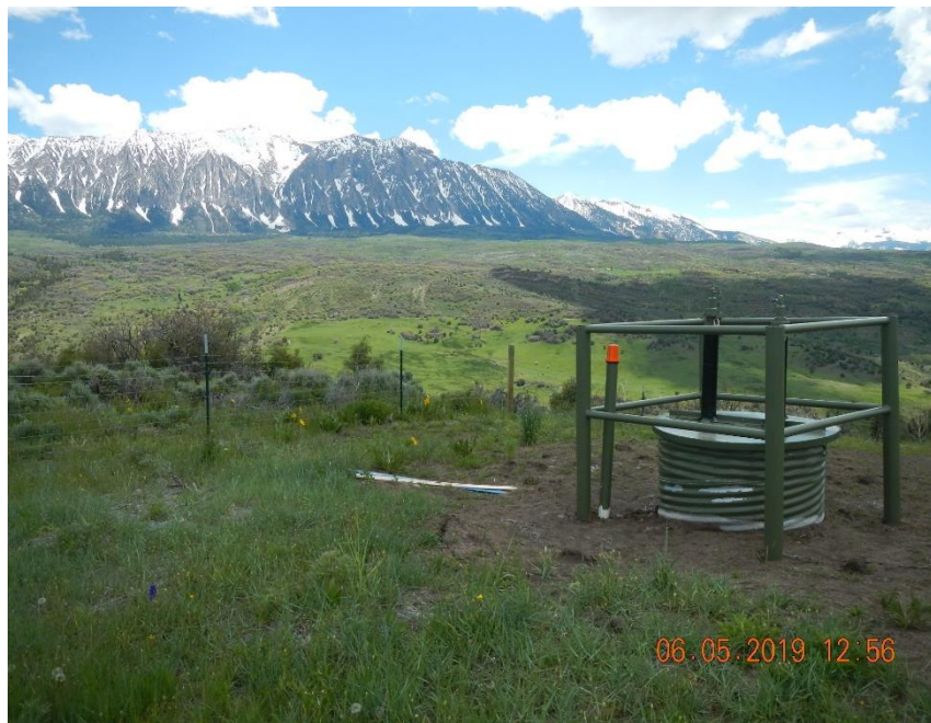
Valve can with vent valve risers for gas and produced water gathering lines.
