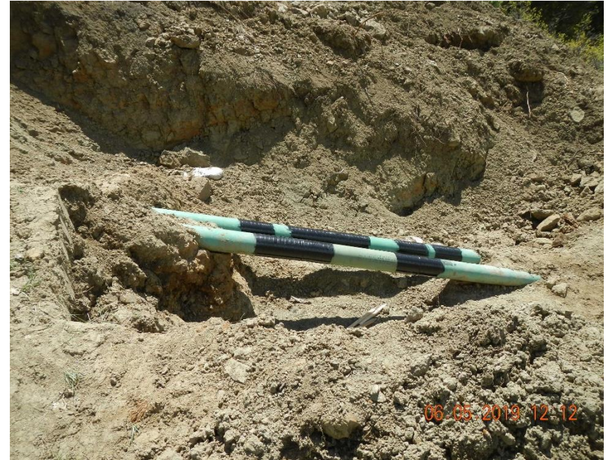
Gathering lines from Hotchkiss Federal #20-12D. Produced water gathering line is the closest pipe.
