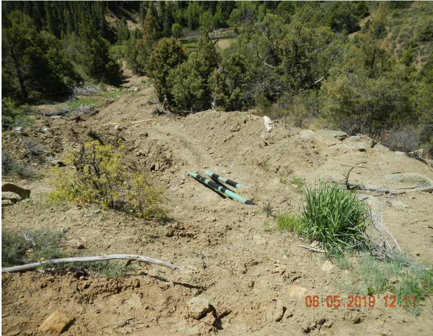
Spill/Release Point ID #464354. Gathering lines exposed in open excavation during this inspection.
