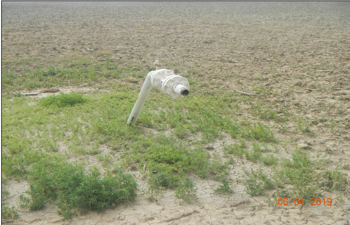
Photo 2. A pipe riser remains at the location. Interfering with farming operations.
