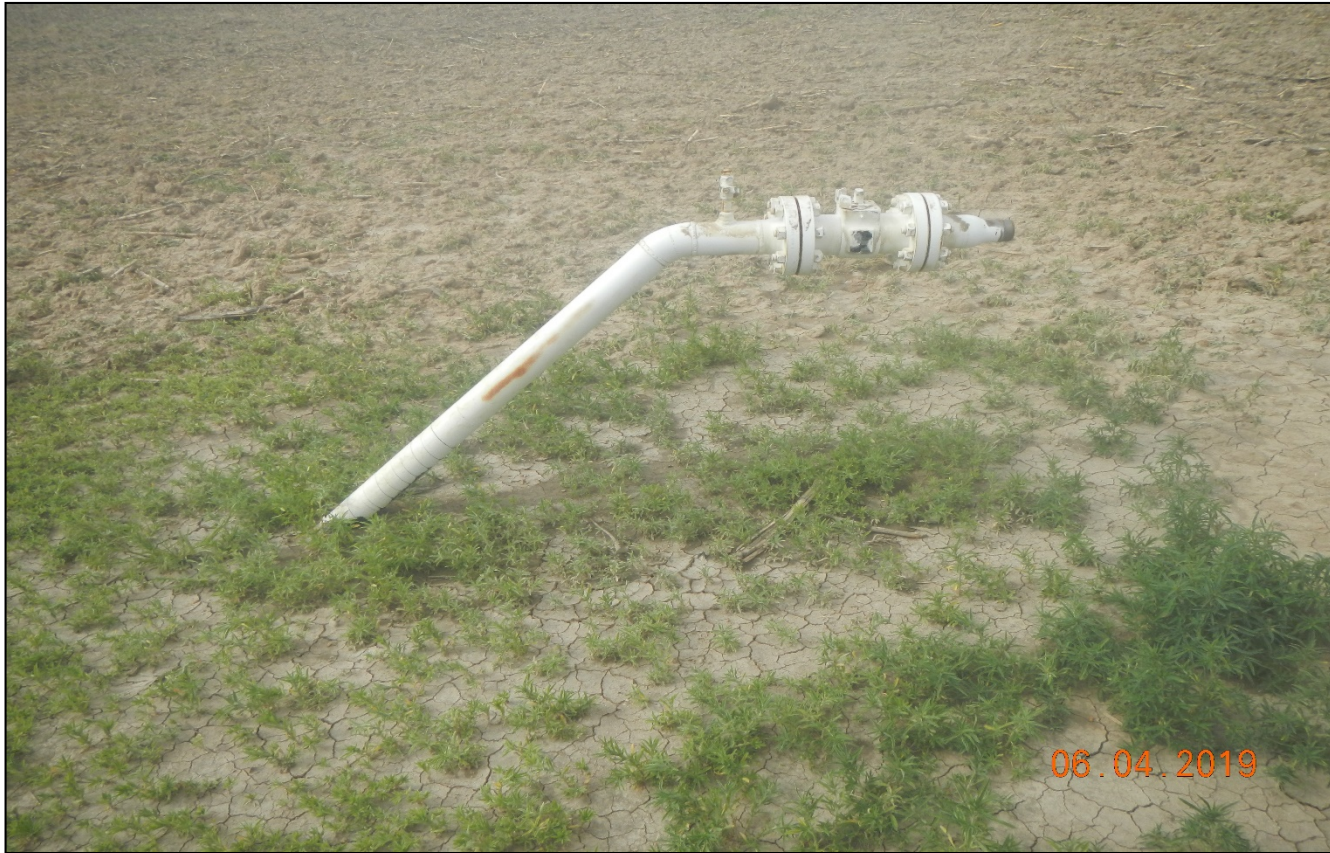
Photo 1. A pipe riser remains at the location. Interfering with farming operations.
