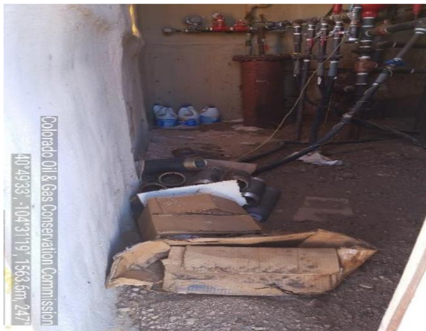
Photo 5 – Trash in Heater Treater house from previous inspection Doc ID 679600271
