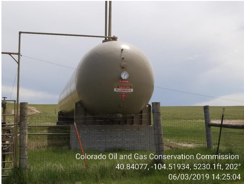
Photo 5 – 36,000 gallon Natural Gas Tank
