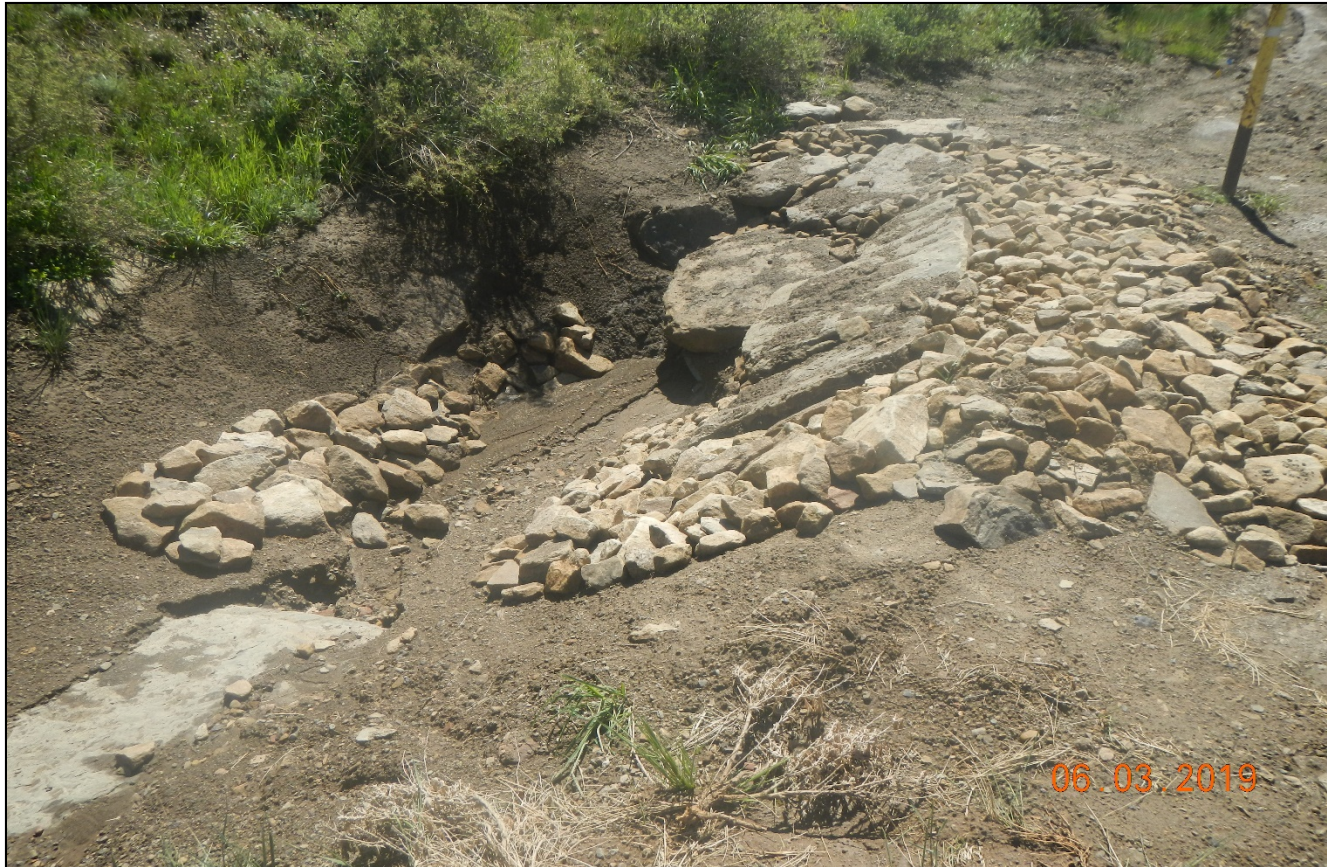
Photo 5. Culvert was repaired however, sediment is already filling up the culvert. Check dams may need to be installed up the road further.
