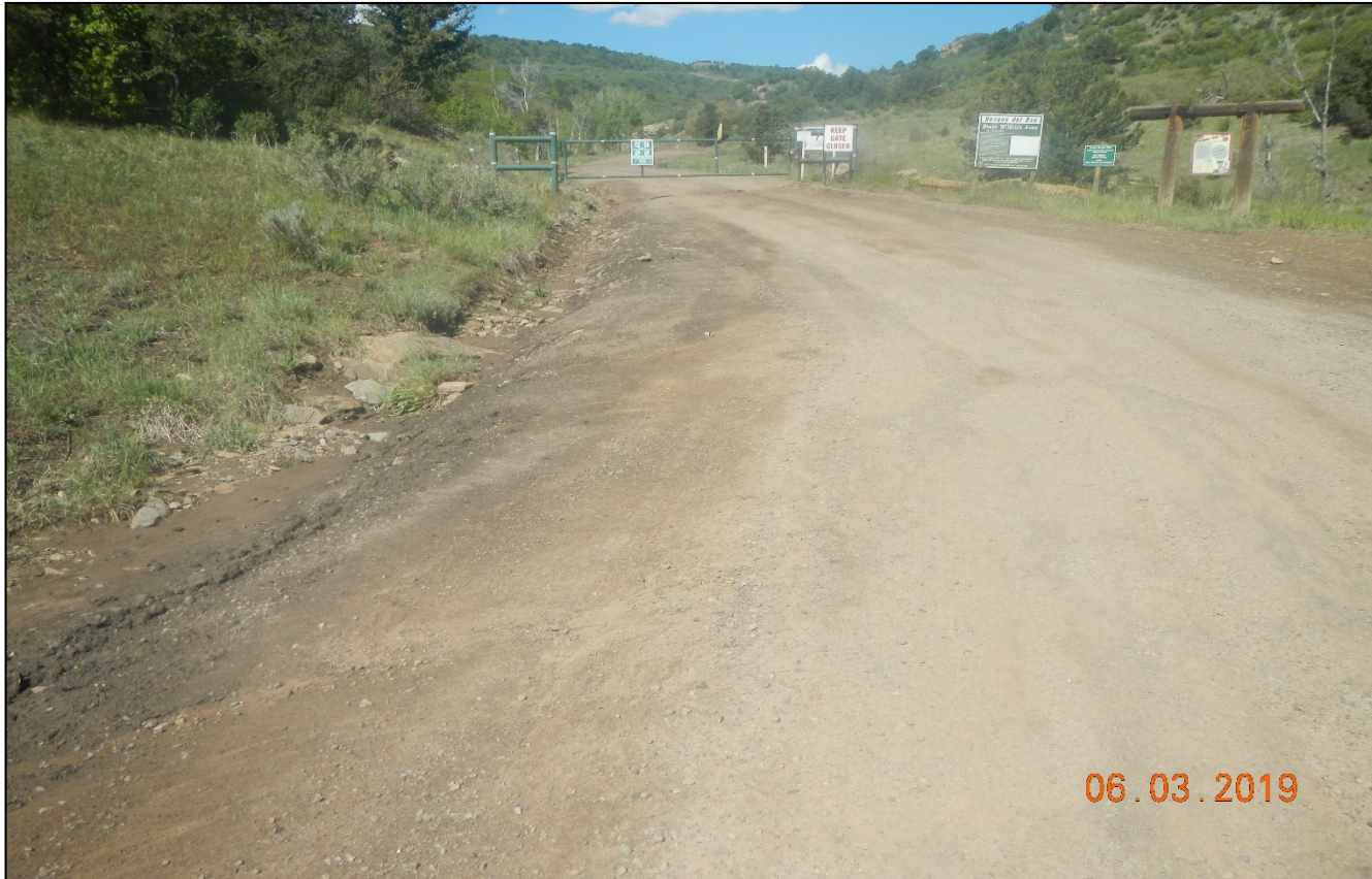
Photo 2. Facing northwest along the main road at the gate of Cherry canyon. Erosion issues have been repaired in this area.
