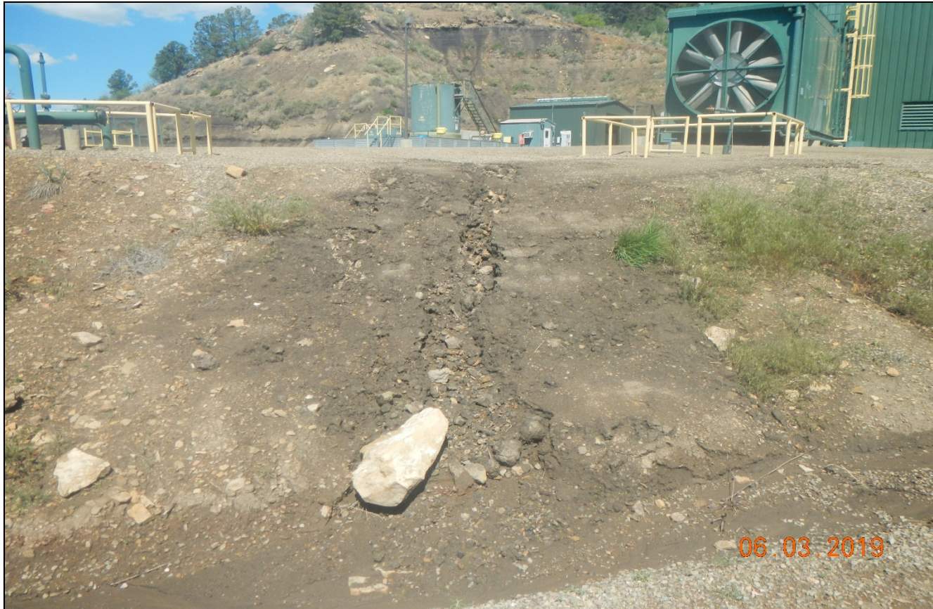
Photo 7. There is still erosion issues at the east side of the pad.
