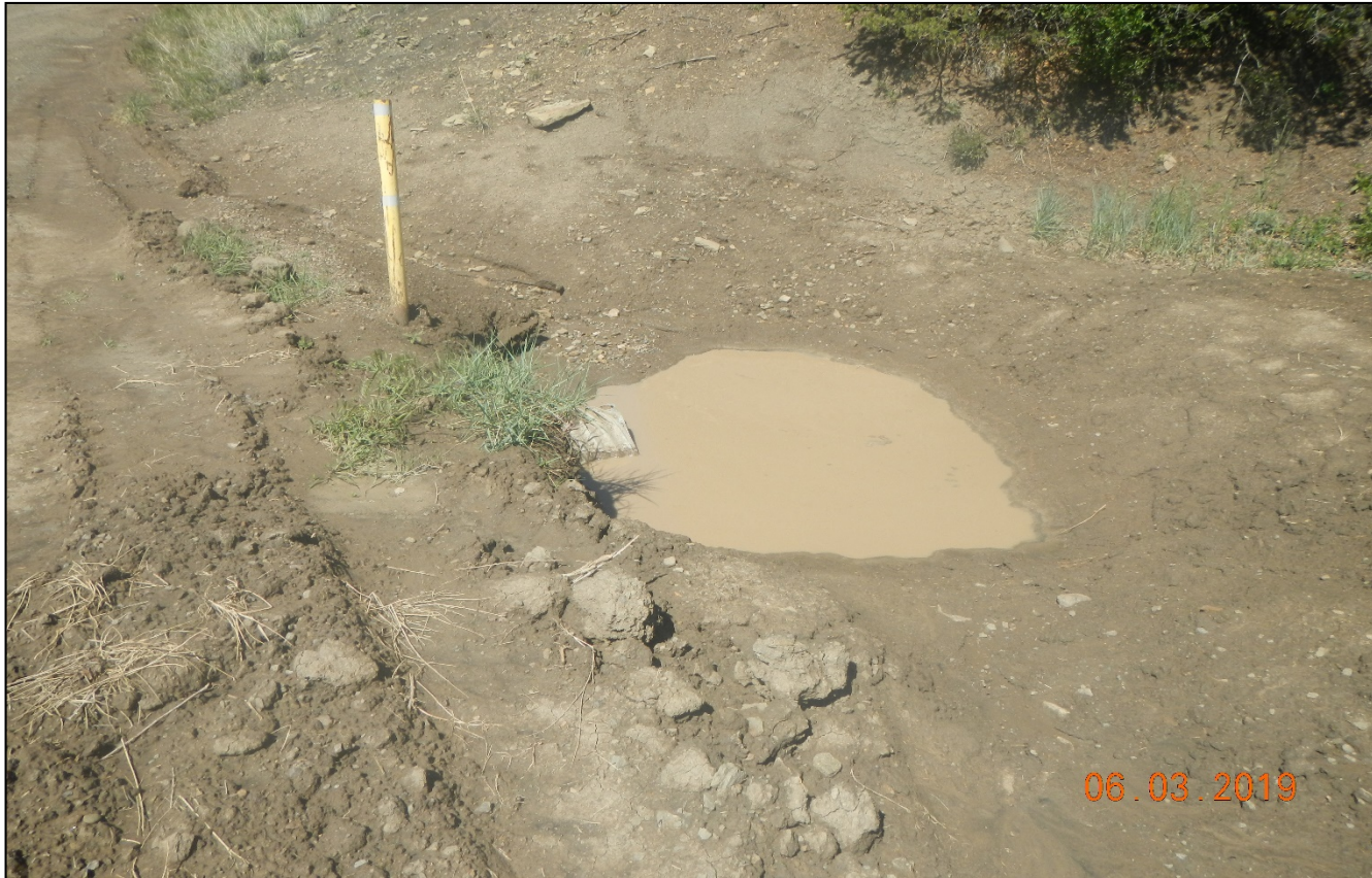
Photo 4. Culvert up the road has been cleaned out. Water shown in the photo is not draining well thru the culvert. This may create issues in the future.
