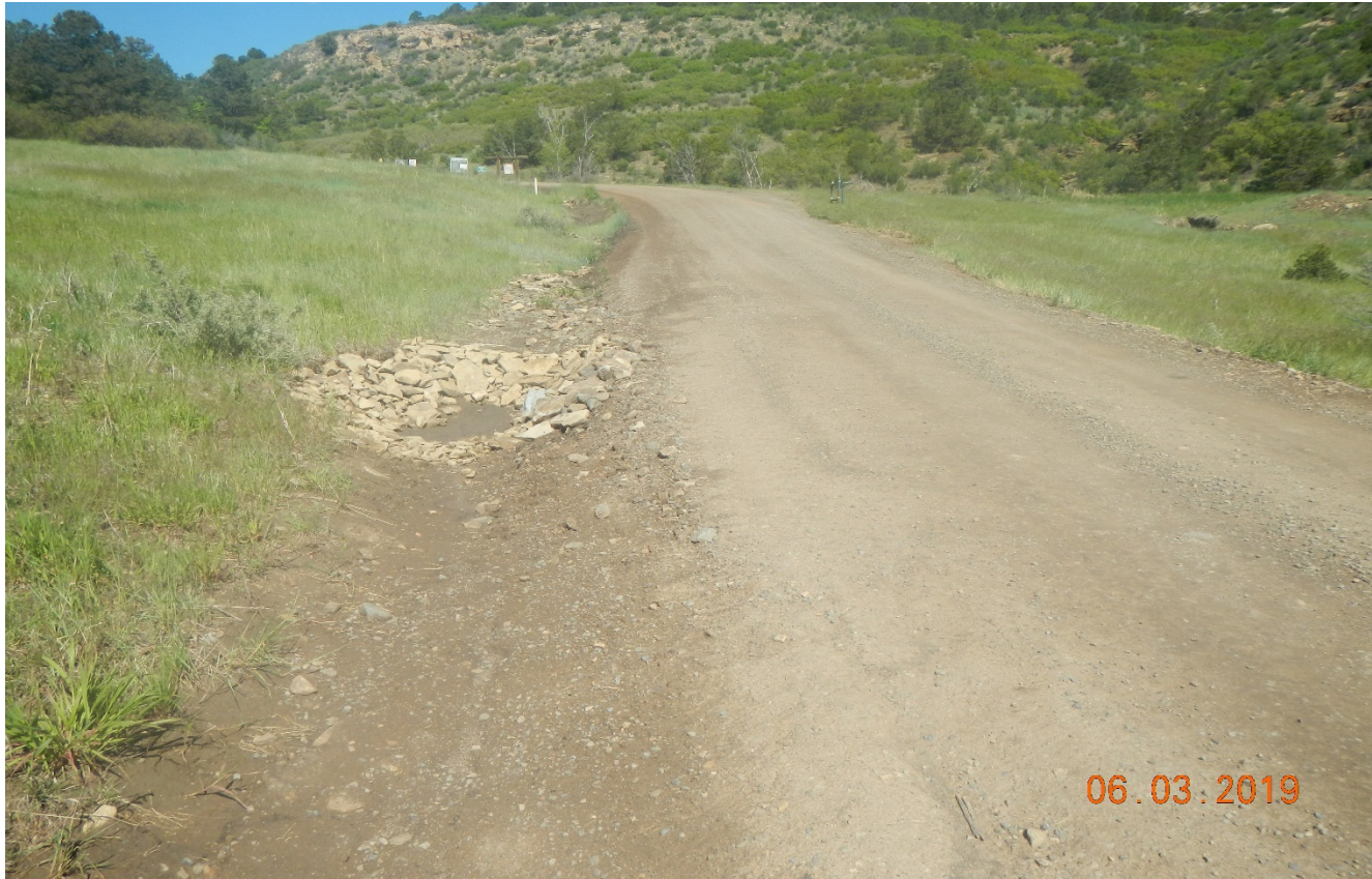
Photo 1. Facing west along the main road near the gate of Cherry canyon. Erosion issues have been repaired in this area.
