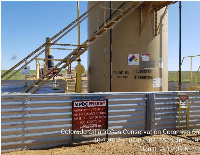
Photo 1: Centralized Tank Battery
