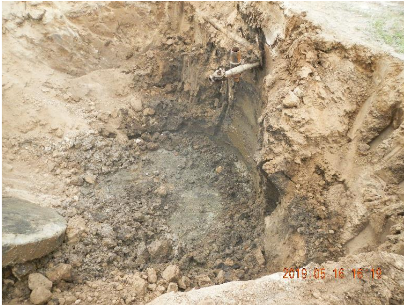
Photo 11: Concrete sump broken up and removed. Flow lines sticking out of dirt wall.
