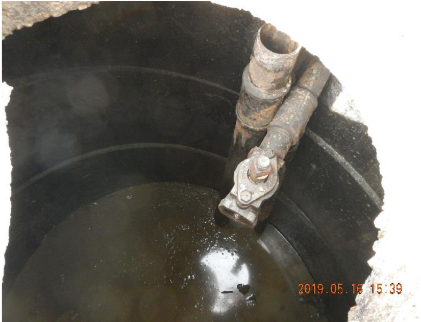
Photo 9: Flow lines inside concrete sump.
