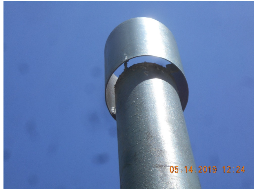
Separator vent with no bird screen.
