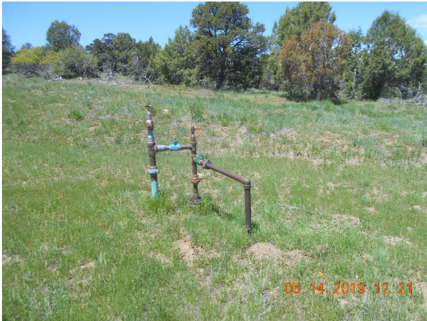
Riser for off location gathering line.
