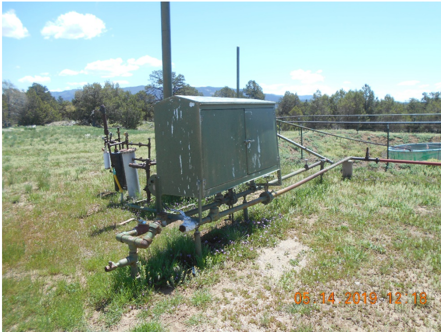
Disconnected and unused flowline on W side of meter housing needs removal
