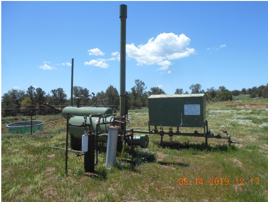
Separator, meter housing and domestic taps.
