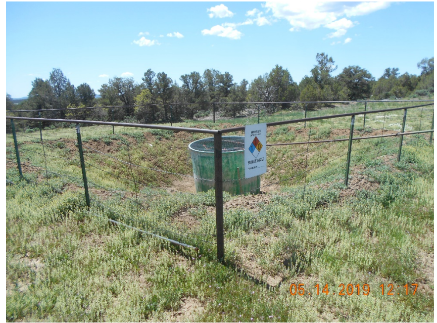
Blowdown tank with fencing and sign.
