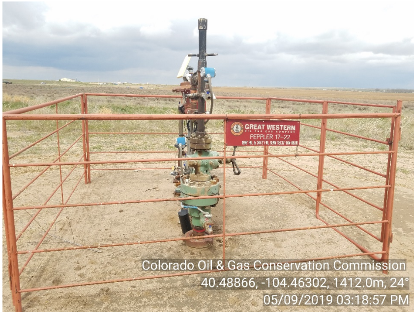
Photo #1 Peppler 17-22 (05-123-25817) Wellsite Shut-In | SI Emergency Number NOT posted from prior insp
