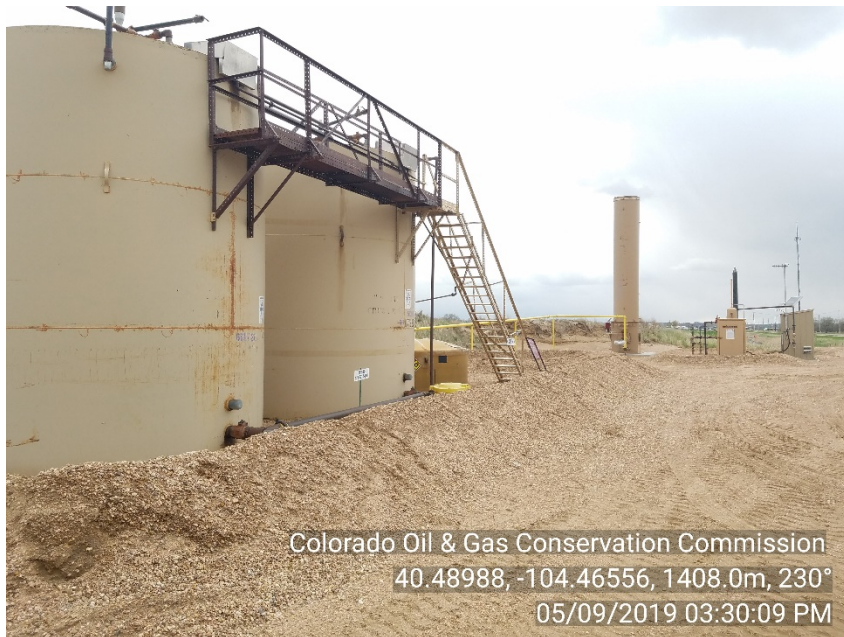
Photo #3 Peppler 17-12, 17-22 Battery Shut-down Illegible capacity – Condensate tanks from prior insp.
