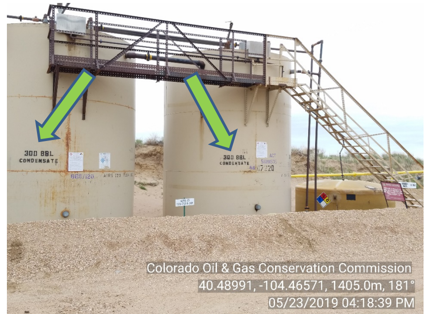
Photo #4 Peppler 17-12, 17-22 Battery Shut-down Condensate tanks – Capacity NOW Legible
