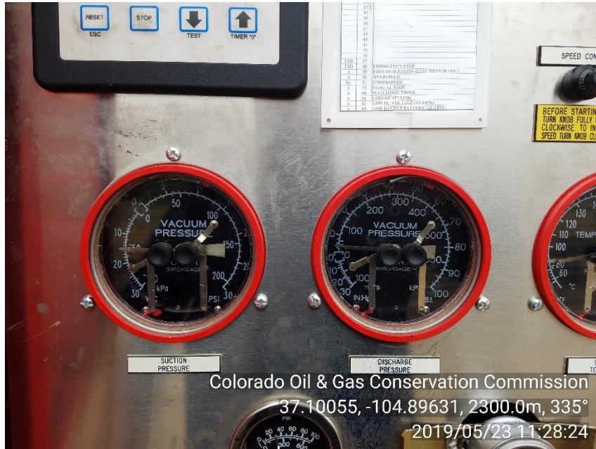
PHOTO 3: Vacuum pump observed on well without COGCC approval. Provide COGCC with documentation showing approval of use of vacuum pump. CA DATE 6/8/19
