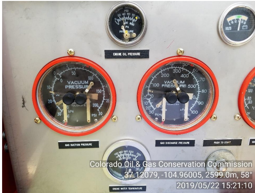
PHOTO 3: Vacuum pump observed on well without COGCC approval. Provide COGCC with documentation showing approval of use of vacuum pump. CA DATE 6/7/19.
