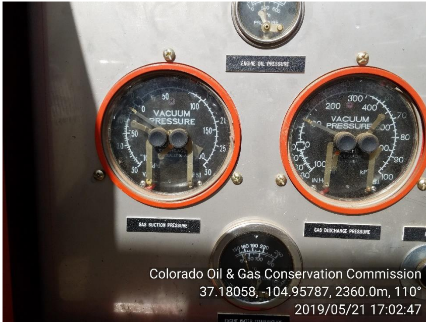
PHOTO 3: Vacuum pump observed on well without COGCC approval. Provide COGCC with documentation showing approval of use of vacuum pump. CA DATE 6/5/19
