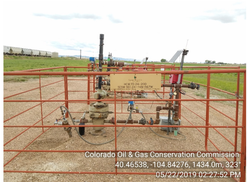
Photo #2 HCW FD 24-20D Wellsite Shut-In | SI Correct sign NOW posted Well name NOW correct
