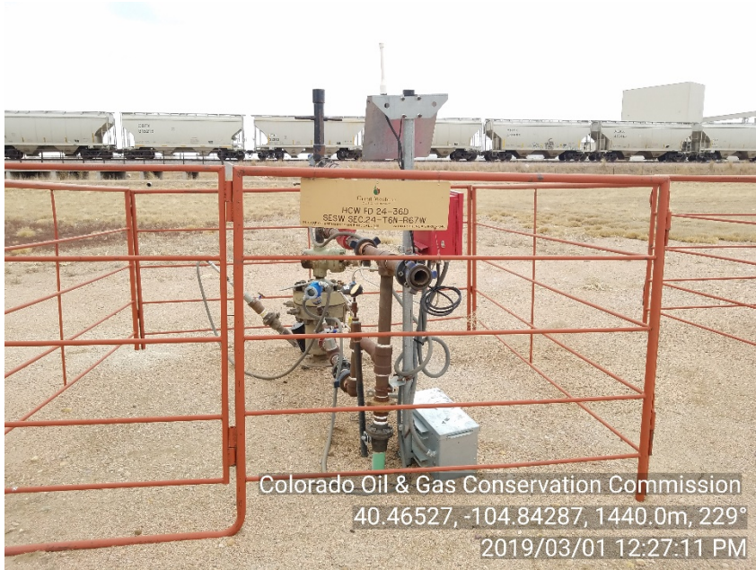
Photo #1 HCW FD 24-20D (05-123-35598) Wellsite Shut-In | SI Incorrect sign posted Well name incorrect from prior insp.
