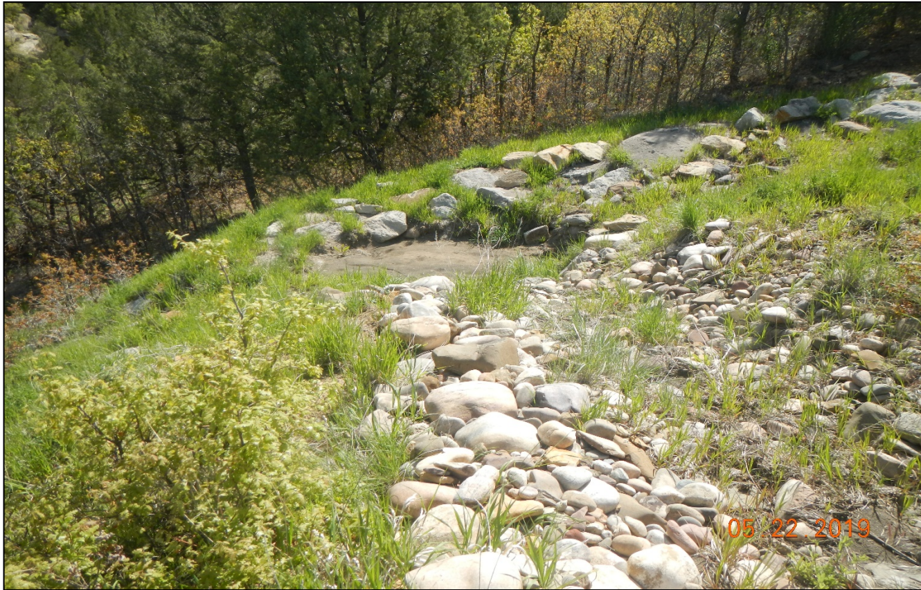
Photo 6. The sediment trap at the east side of the location needs to be cleaned out.
