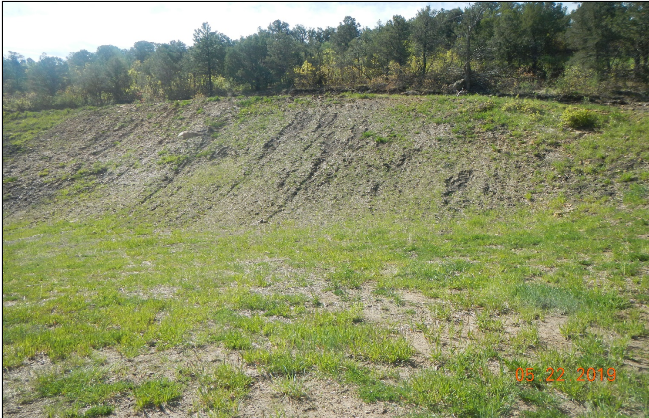
Photo 2. Facing toward the cut slope which appears to have recently been seeded and mulched. There is some rilling occurring,
