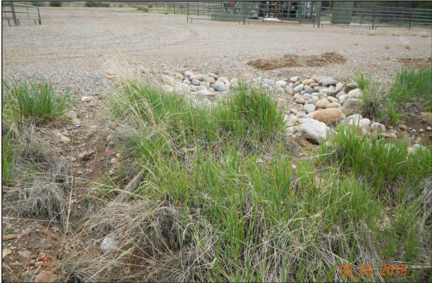
Photo 2. View of erosional side-channel forming within the western project area, adjacent to the cobble run-down.
