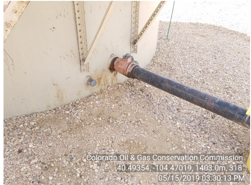
Photo #6 Cornish 17-11 Condensate tank Stained soil at loadout – appears remediated
