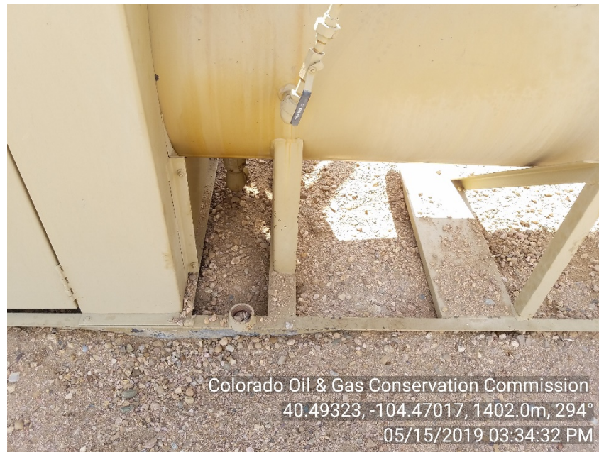
Photo #8 Cornish 17-11 Separator Stained soil – appears remediated
