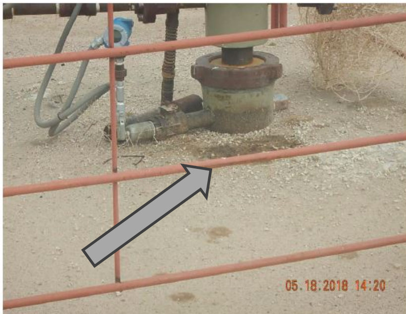
Photo #3 Cornish 17-11 Wellsite Stained soil from prior insp.
