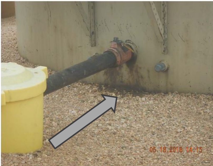
Photo #5 Cornish 17-11 Condensate tank Stained soil at loadout from prior insp.
