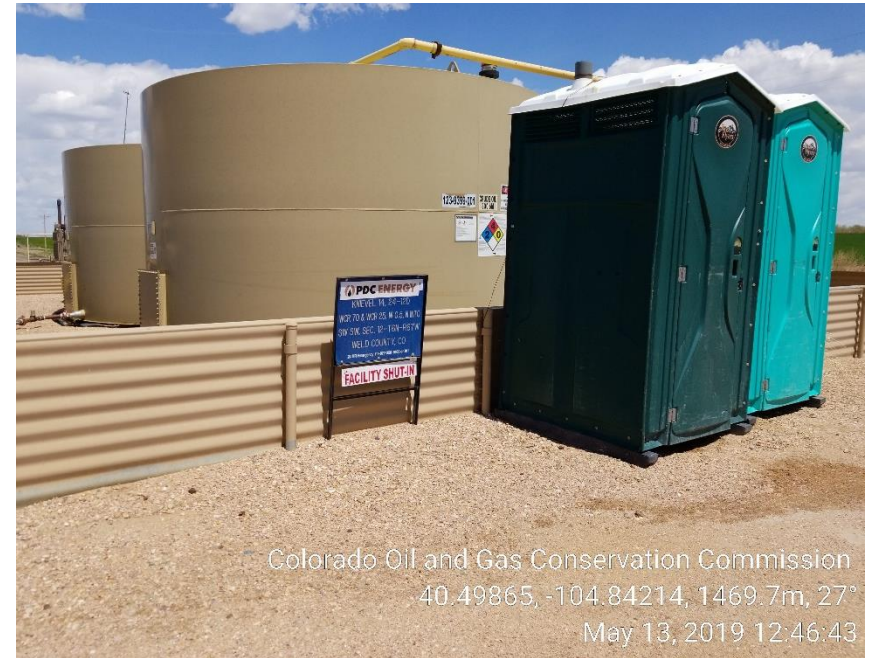
Photo 2: Centralized Tank Battery
