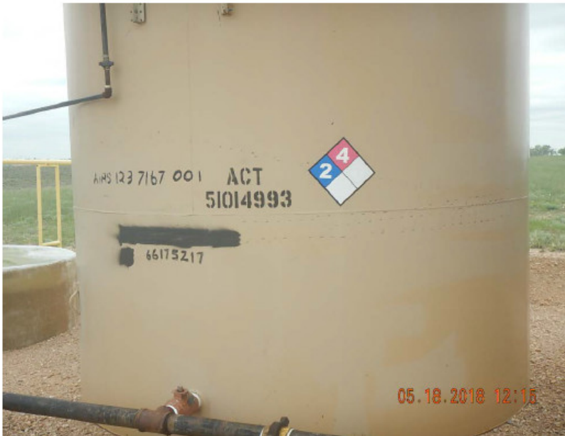
Photo #7 Cache 17-52, 17-21 Battery West Prod Tank – Contents-Capacity NOT posted from prior FIR
