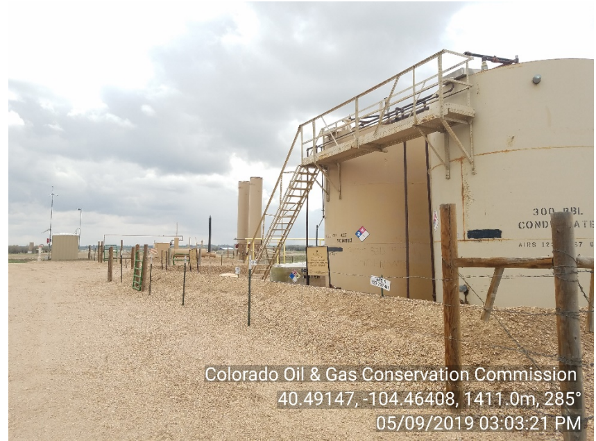
Photo #2 Cache 17-52, 17-21 Battery Shut-down
