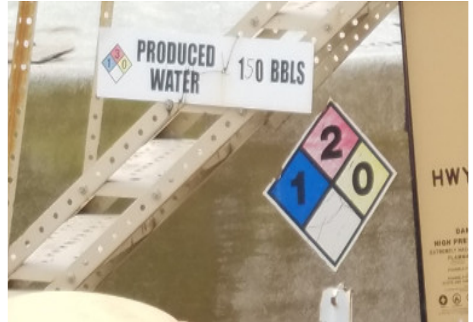
Photo #6 Cache 17-52, 17-21 Battery Produced H2O vault– Correct Capacity posted
