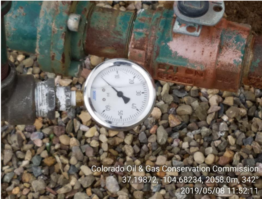
PHOTO 5: TUBING PRESSURE 0 THROUGHOUT THE TEST.
