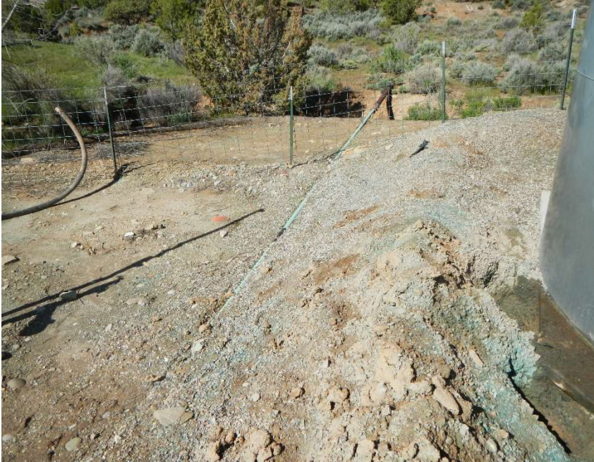
Photo #3 – Compromised tank battery with the two excavations and the arroyo (south, ~42 feet)
