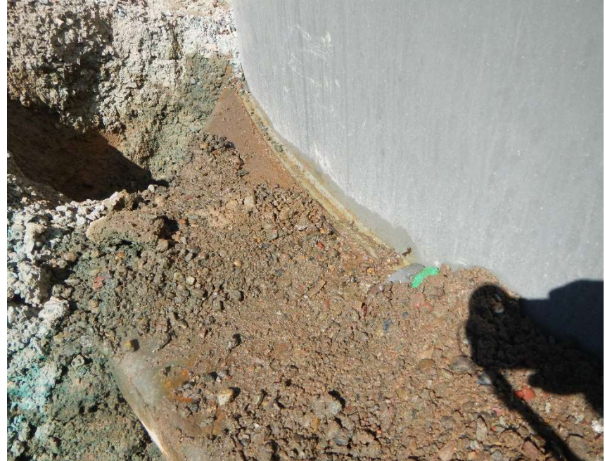
Photo #4 – A 1” stick plugging pin hole sized leak. Excavations to the south of the leak. Oily stained soil located beneath the leak.
