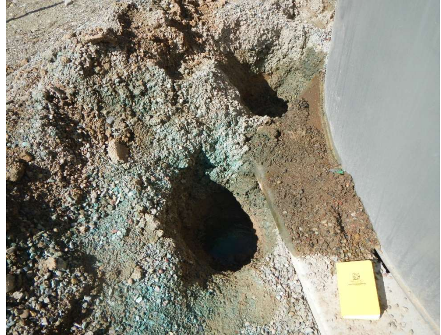
Photo #2 – Two Excavations south of the leak, oily stained sidewalls.
