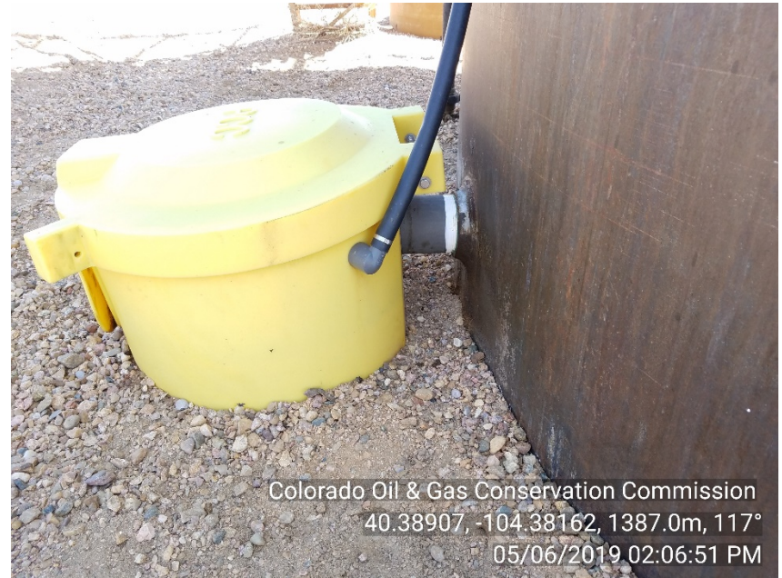
Photo #4 Monahan Federal #24 Battery Crude Oil tank load out Stained soil, prior seepage Appears Mitigated
