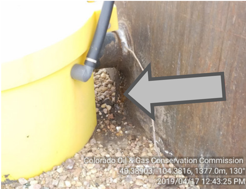
Photo #3 Monahan Federal #24 Battery Crude Oil tank load out Stained soil, prior seepage from prior FIR
