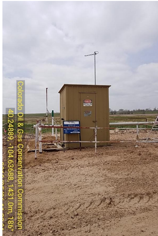
Photo 2 Gas Meter Run Remaining on Location
