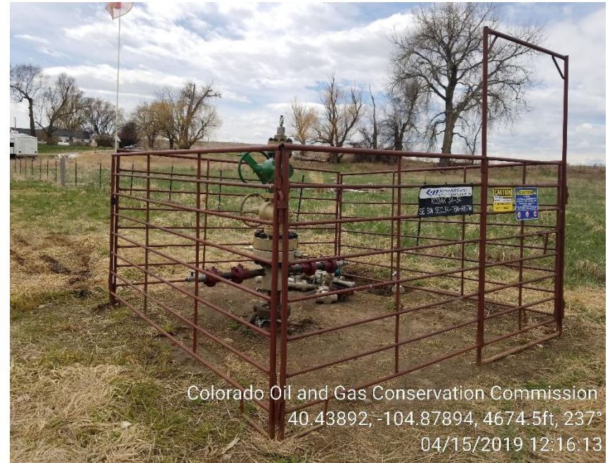
Photo 2 – Wellhead, well SI at the time of inspection
