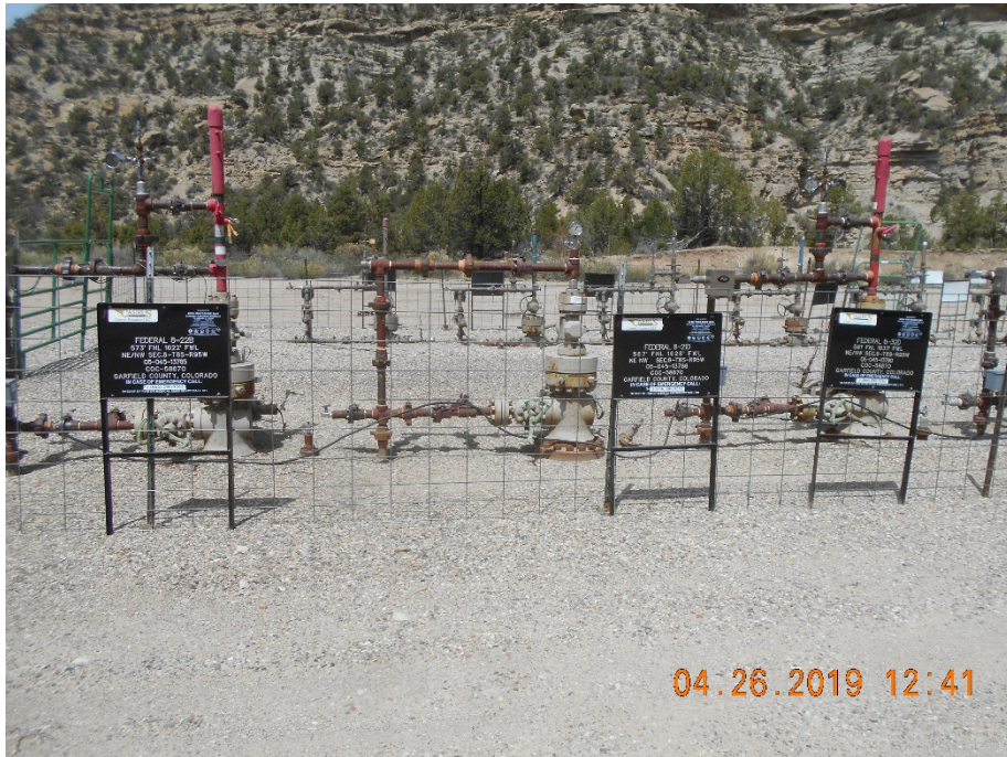
Wellheads with fencing
