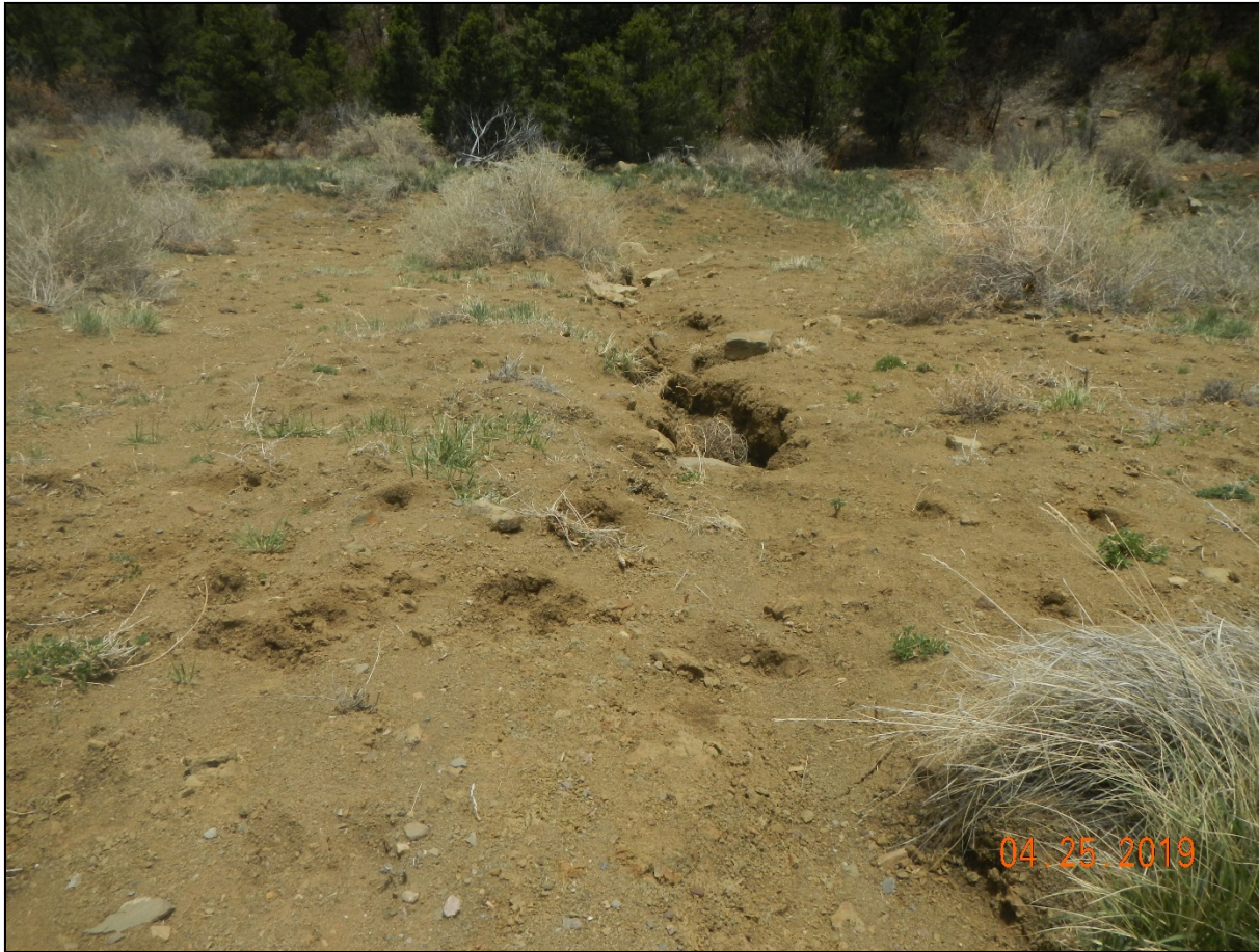
Photo 3. There is an erosion channel that formed at the south fill slope.
