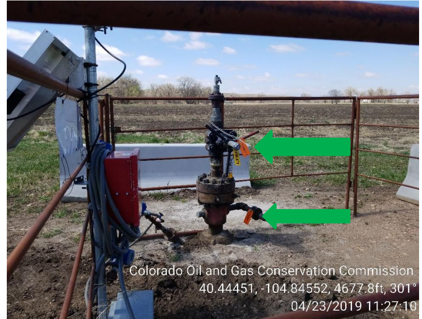
Photo 2 – Wellhead now has the Orange Decommission Tag installed.
