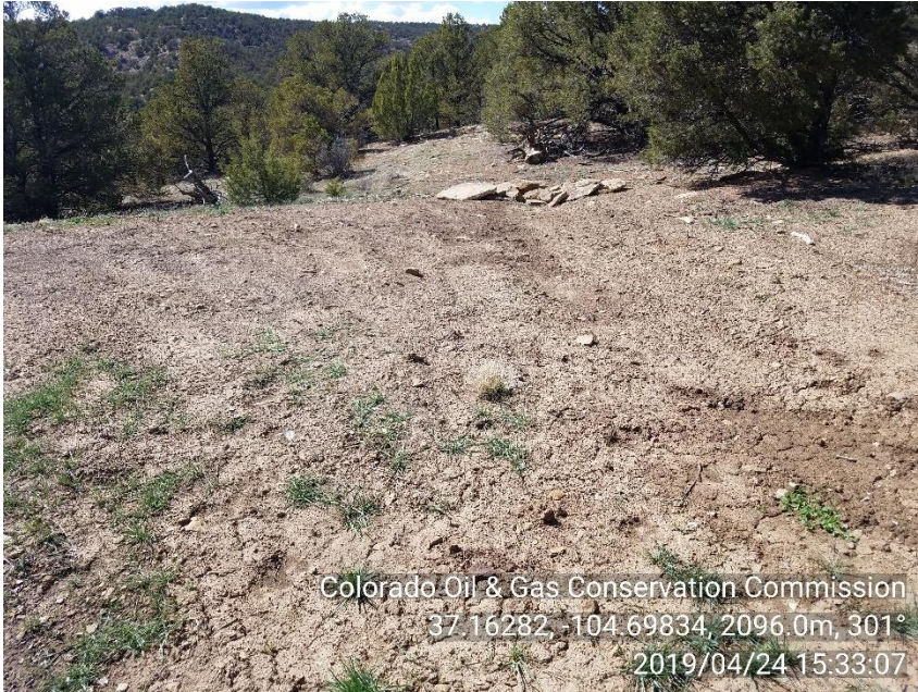
PHOTO 5: INADIQUATE VEGETATION COVER ON WEST SIDE OF LOCATION
