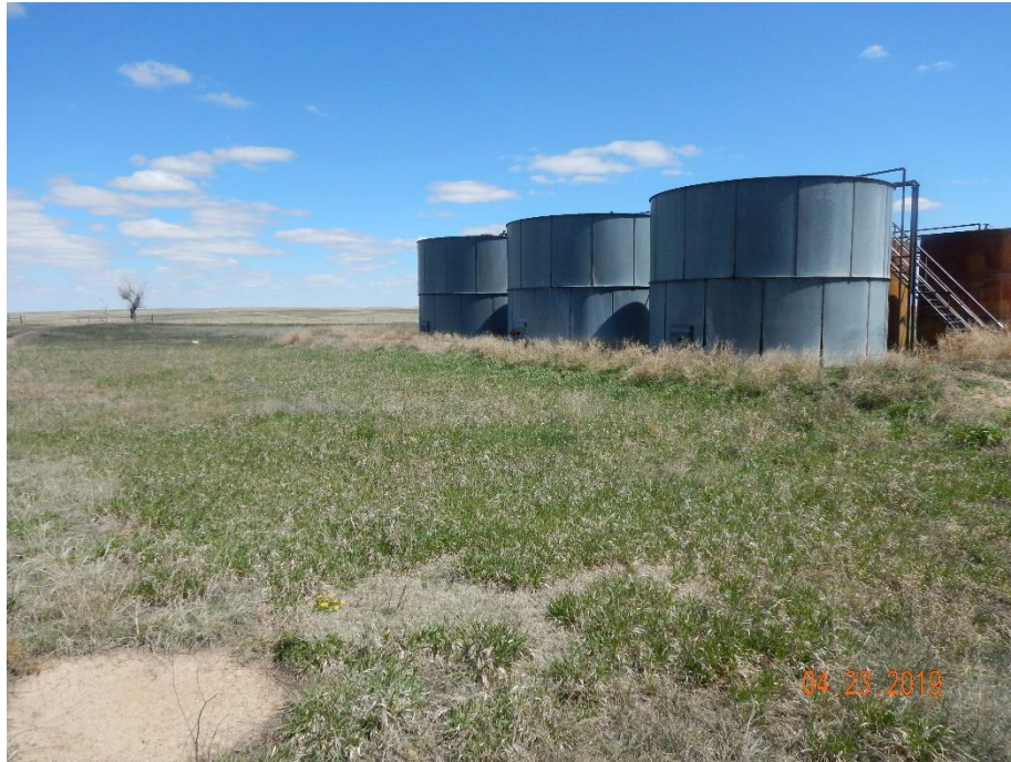
Photo 1: Photo taken from the southwest end of the tank battery, facing north. Photo shows weed debris accumulation on the berms and around equipment.
