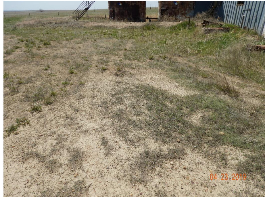
Photo 6: Photo shows undesirable weedy plant establishment, and weed debris accumulation on berms and equipment.
