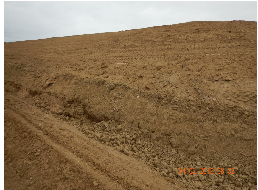
Photo 2. Photo taken from the southeastern location, facing Northwest. Operator is still in process of constructing the location. The southern fill slope needs to be stabilized and will be tracked in like the eastern fill slope.
