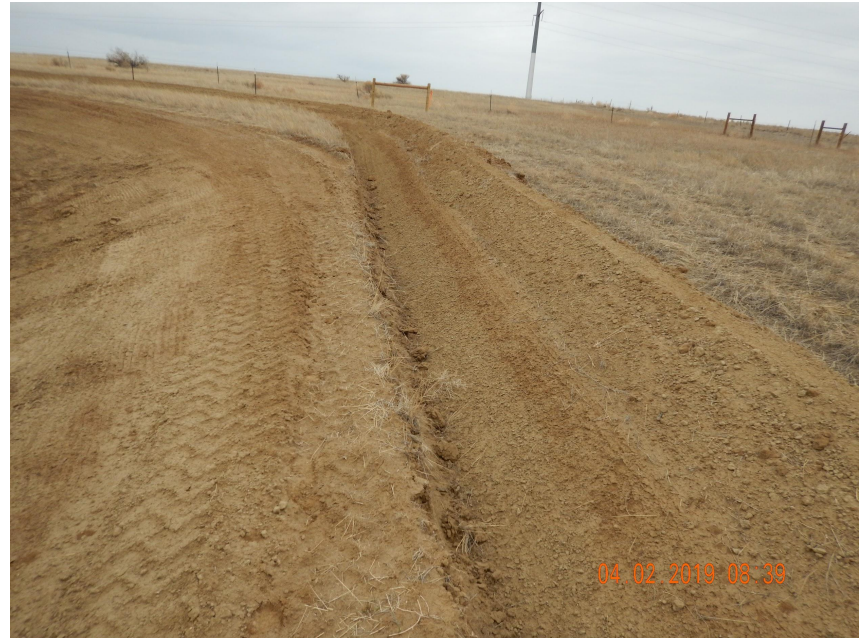
Photo 4. Photo taken from the northwestern location, facing West. Operator shall stabilize the berm BMP, as an unconsolidated berm BMP is not a properly functioning BMP.
