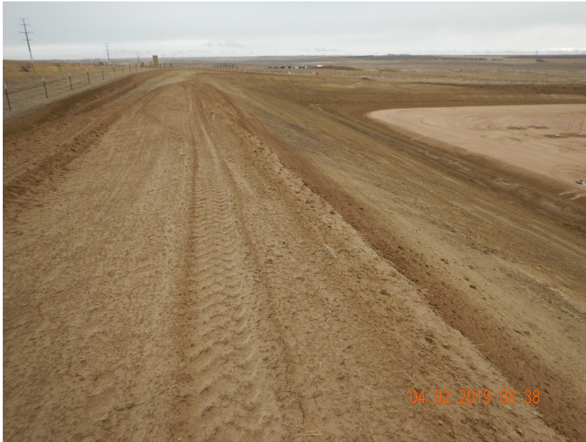
Photo 3. Photo taken from the western location, facing North. Photo illustrates a portion of the topsoil stockpile. Operator shall comply with Rule 1002 to stabilize the topsoil stockpile.
