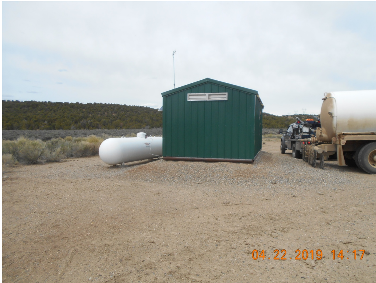
Injection Wellhead inside housing
