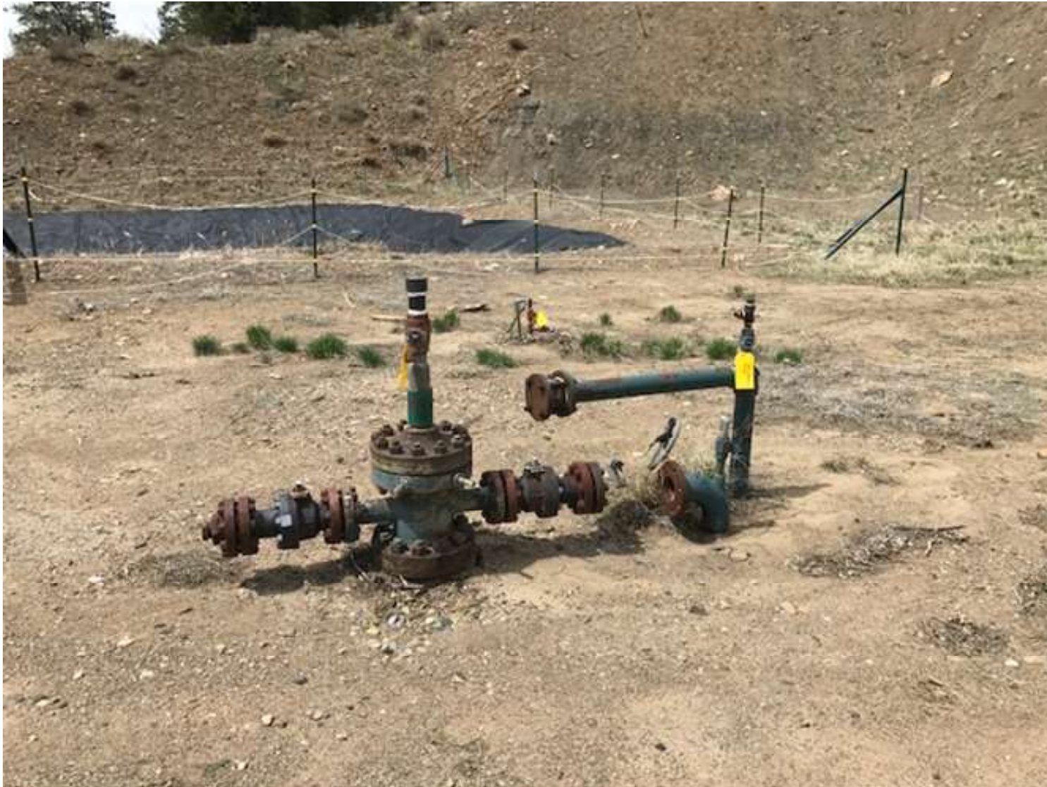
PHOTO 6: THE FLOW LINE RISERS WERE LABELED AND LOTO.
