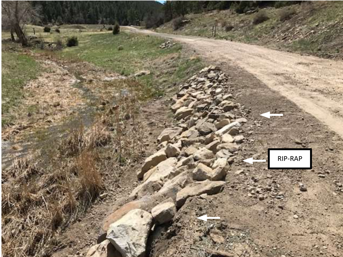
PHOTO 1: THE EROSION OF THE FILL SLOPE ALONG THE MAIN LEASE ROAD TO LOCATION HAS BEEN ADDRESSED. RIP-RAP WAS PLACED ON THE FILL SLOPE FOR SOIL STABILIZATION.
