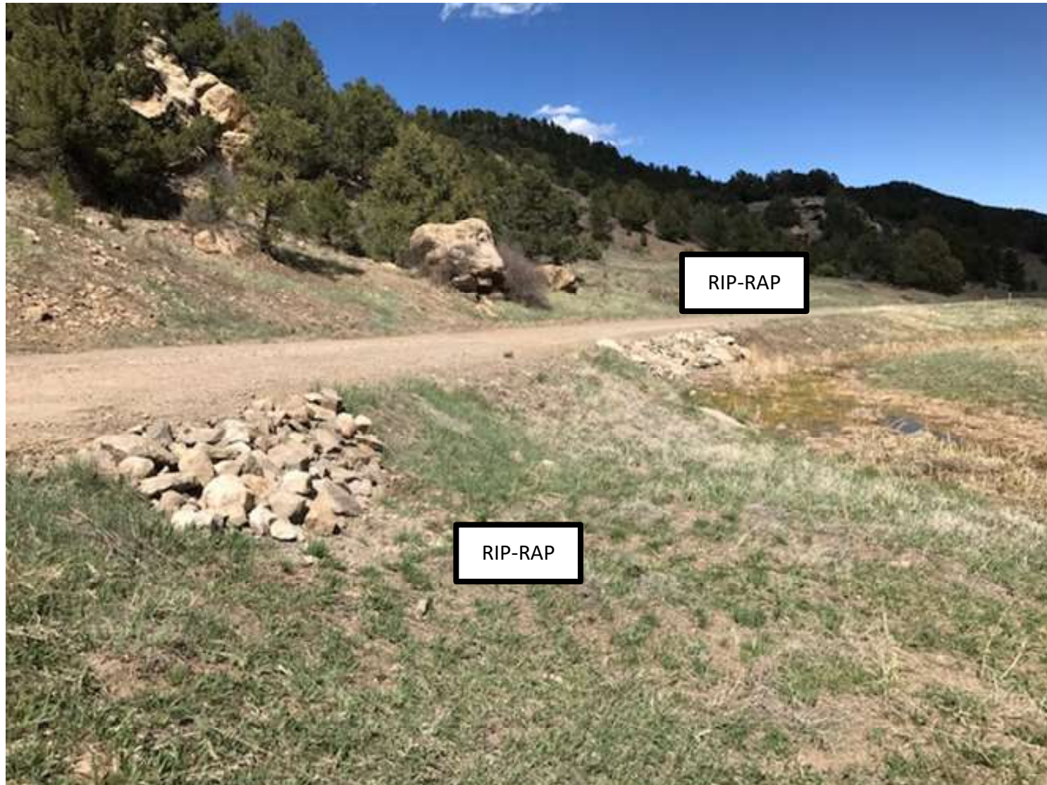
PHOTO 2: THE EROSION OF THE FILL SLOPE ALONG THE MAIN LEASE ROAD TO LOCATION HAS BEEN ADDRESSED. RIP-RAP WAS PLACED ON THE FILL SLOPE FOR SOIL STABILIZATION.
