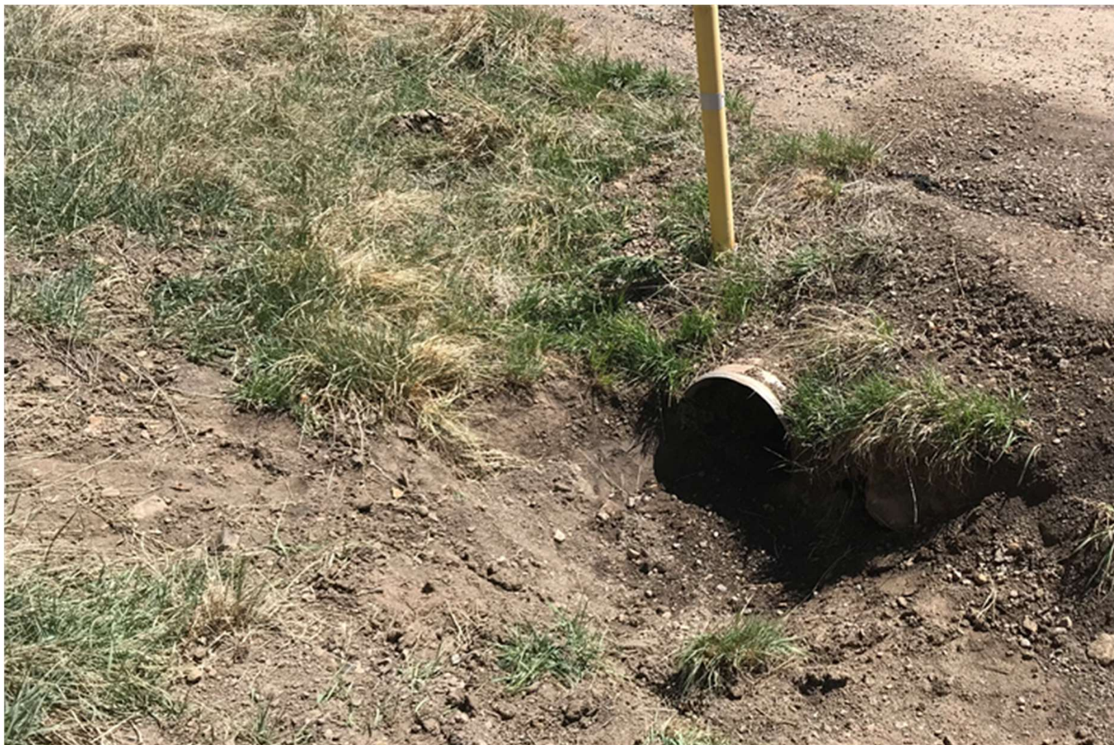
PHOTO 3: THE SEDIMENT WAS REMOVED FROM THE CULVERT INLET TO ALLOW STORMWATER TO FLOW THROUGH CULVERT.
