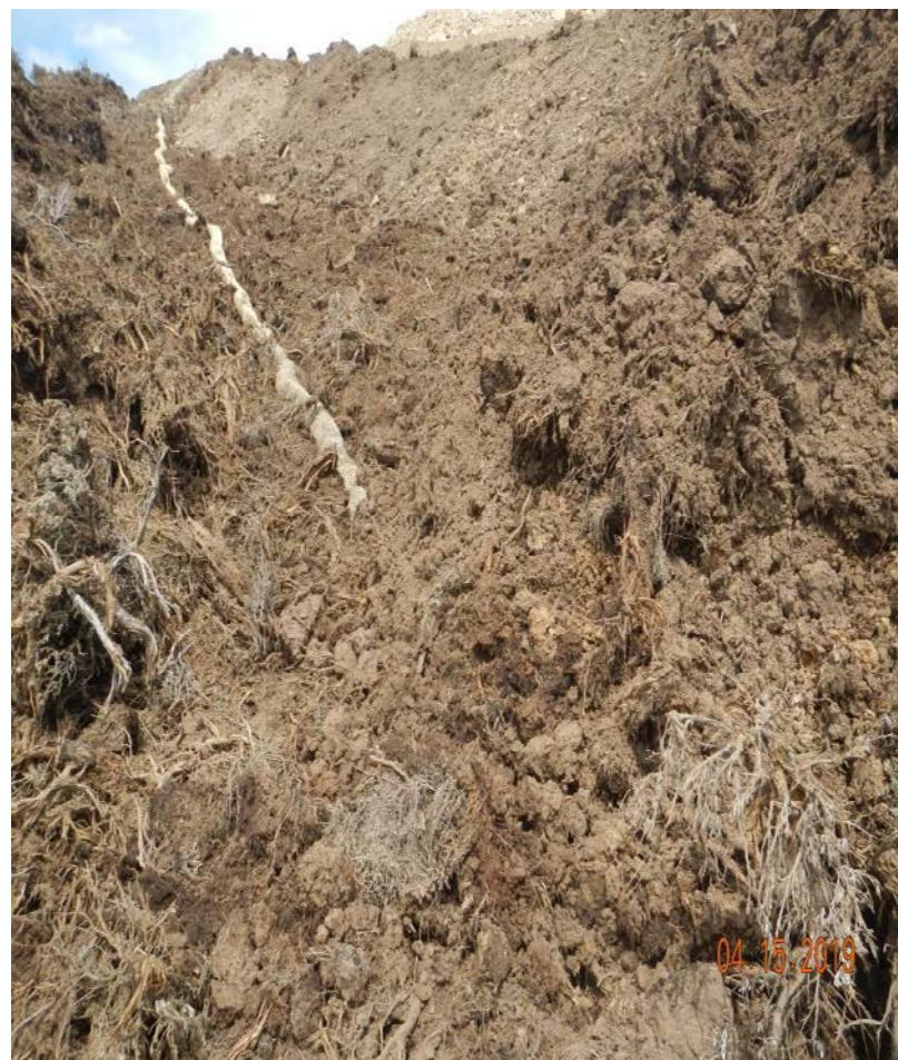
Photo#8: In a few places wattles have been overwhelmed.
