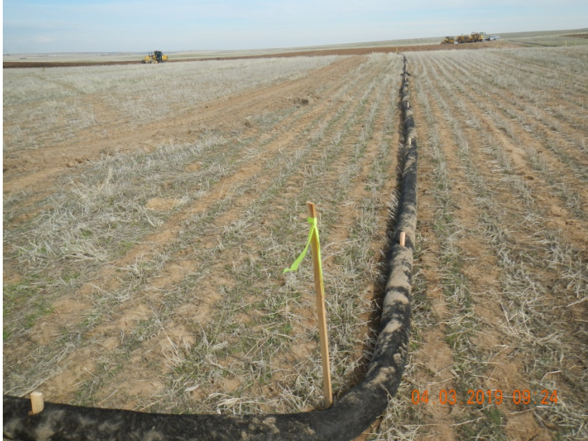
Photo 5. Photo taken from the southeastern perimeter of the location, facing North. Photo illustrates a filtrex BMP that has been installed around the entire perimeter of the location in conjunction with other BMPs.
