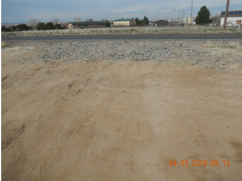
Photo 1. Photo taken from the entrance of the location off Imboden Road , facing West. Appears Operator has installed gravel to potentially limit tracking onto the road.
