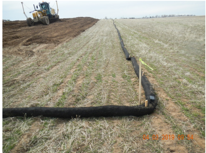
Photo 10. Photo taken from the northwestern perimeter of the location, facing South. Photo depicts the topsoil stock pile that is currently being salvaged.
