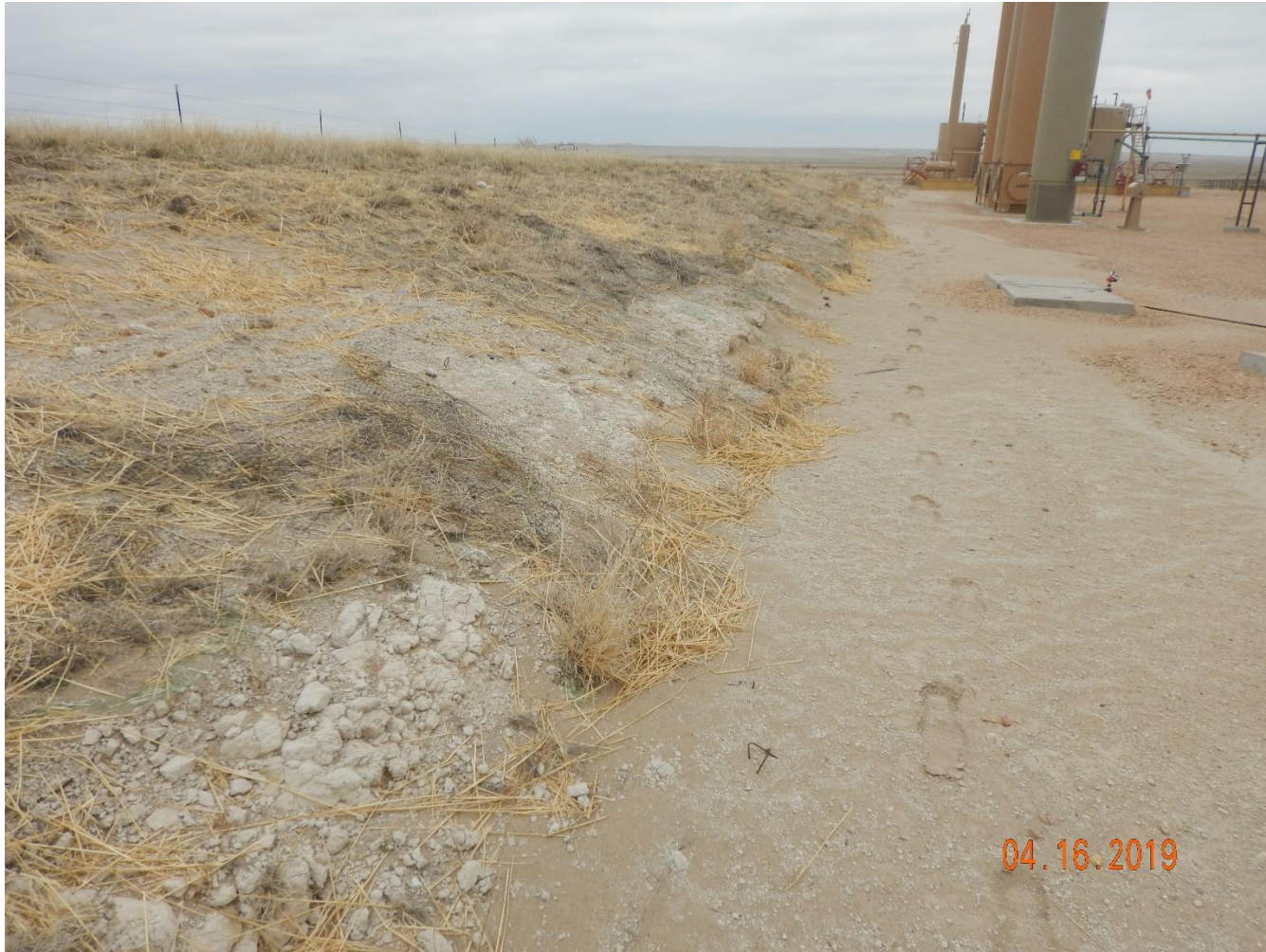
Photo 4: Photo taken from the northwest end of the pad, facing south. Photo shows operator appears to have seeded/mulched slopes on the east.
