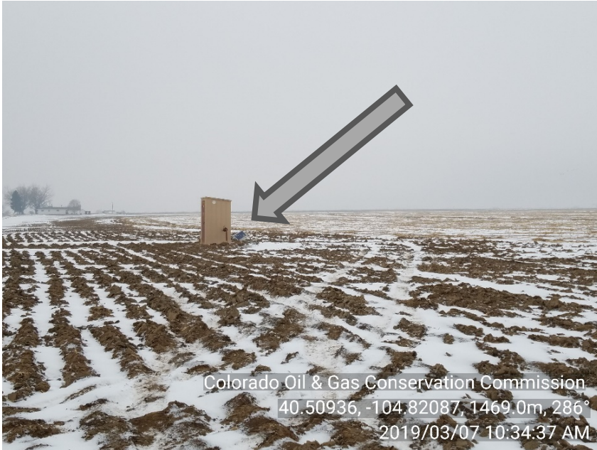
Photo #1 Hergert 1-6 Abandoned Battery site Unused Equipment Gas meter run, Automation tower from prior FIR
