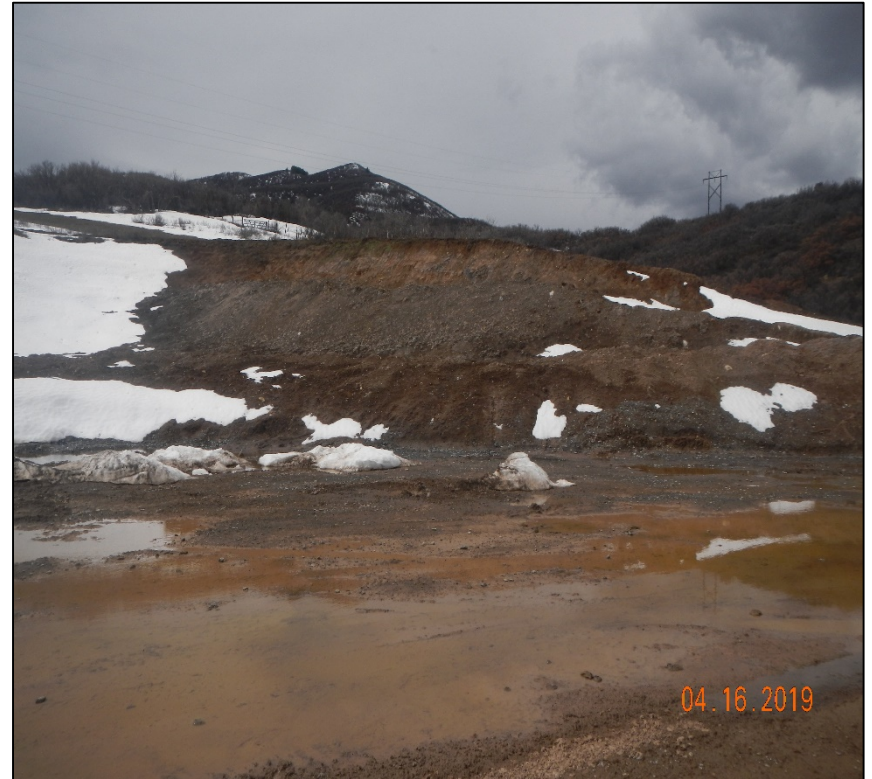
Slope not stabilized
