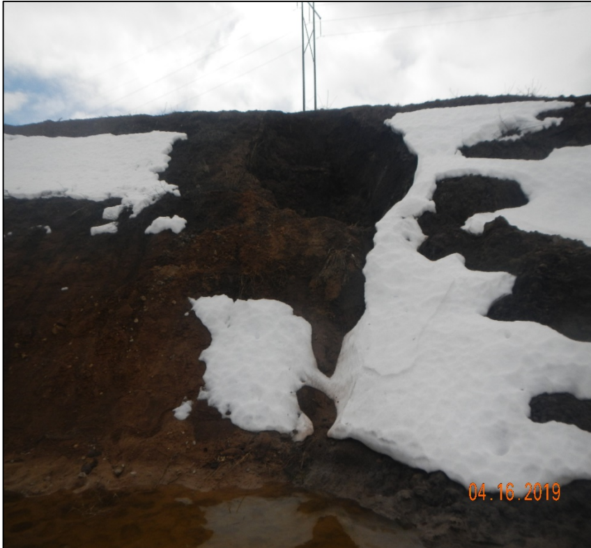
Slope not stabilized
