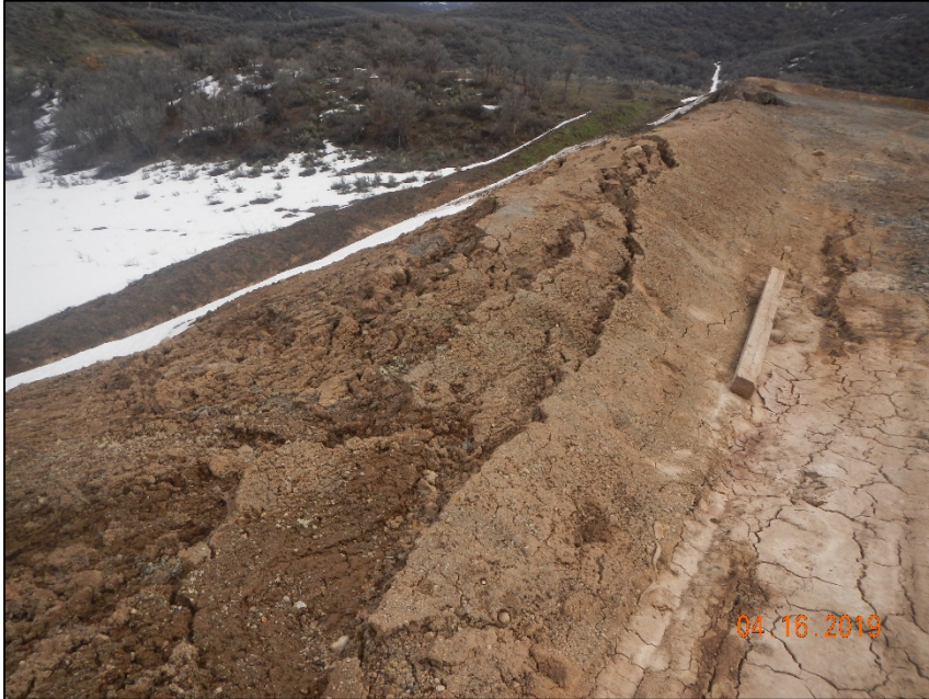
Berm not compacted or stabilized
