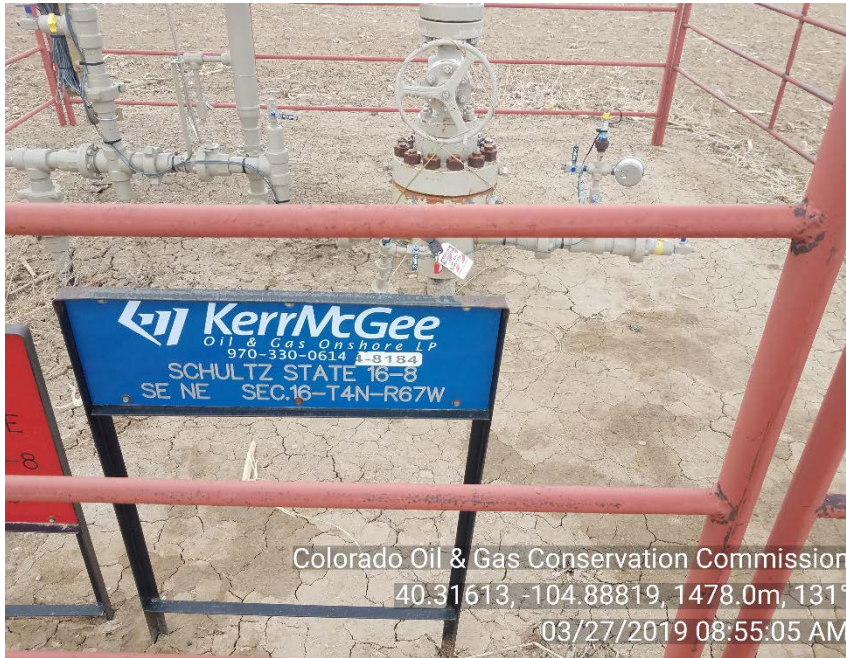
Wellhead sign on 3/27/19
